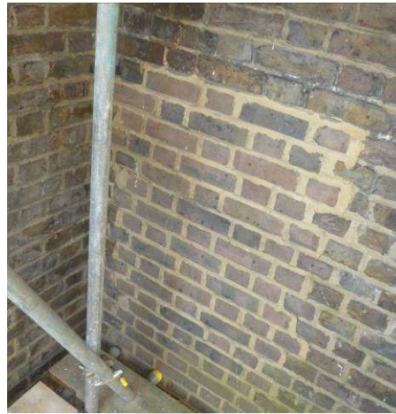
Photo 9: Poor modern repointing.
