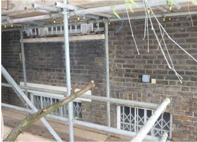
Photo 8: Rear façade with cracking and movement
