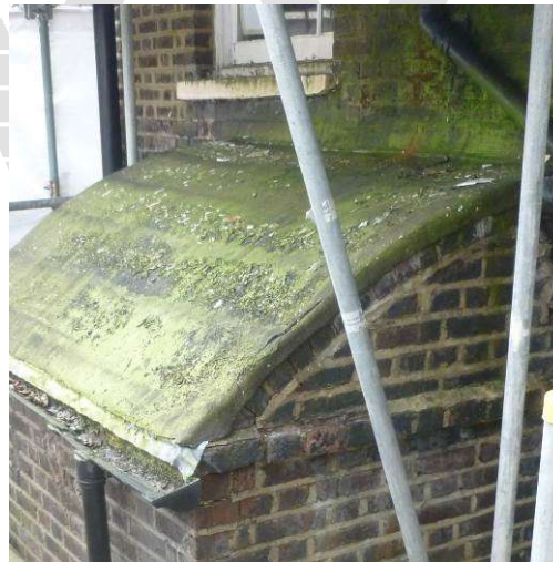
Photo 17: Failed modern asphalt to rear curved roof
