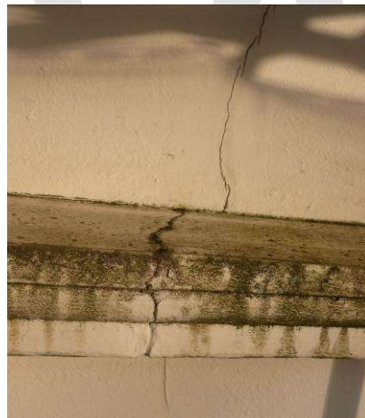
Photo 11: Crack to façade moulding
