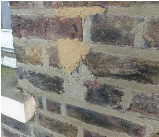
Photo 10: Various poor modern remedial pointing.
