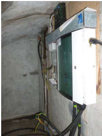
Photo 25: vault with utility supply.
