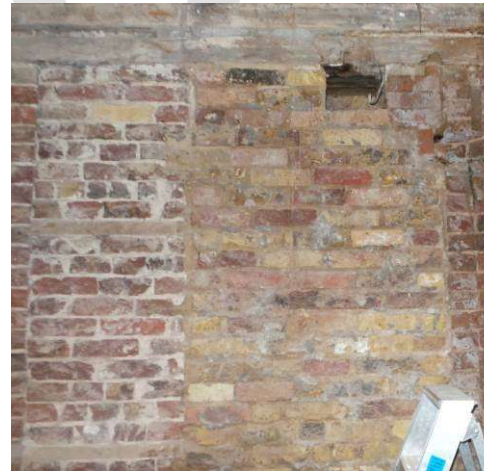
Photo 27: Blocked doorway to inaccessible vault.
