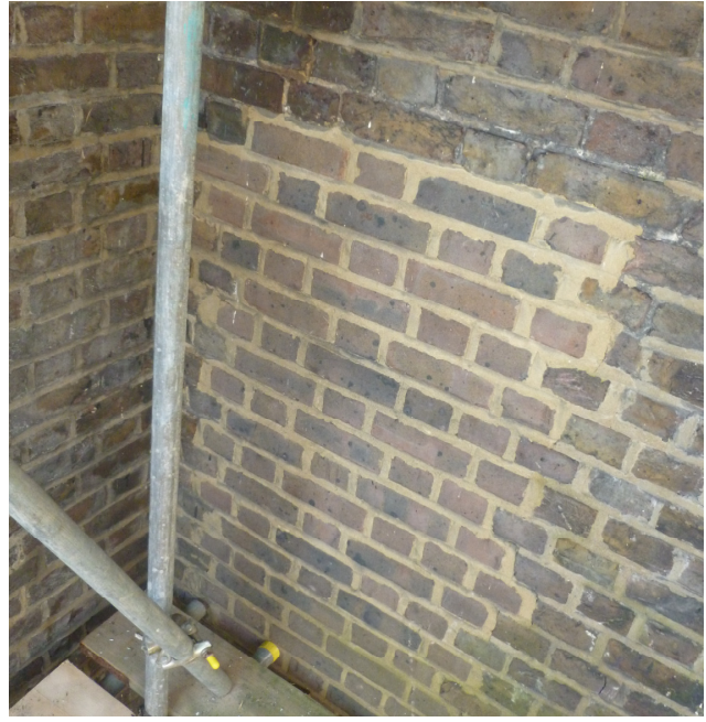
Poor modern repointing previously undertaken.
