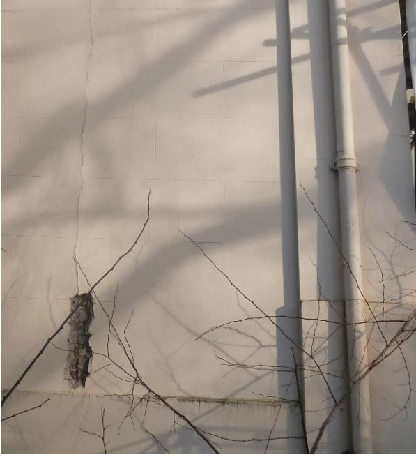
Structural crack running full height of the building.
