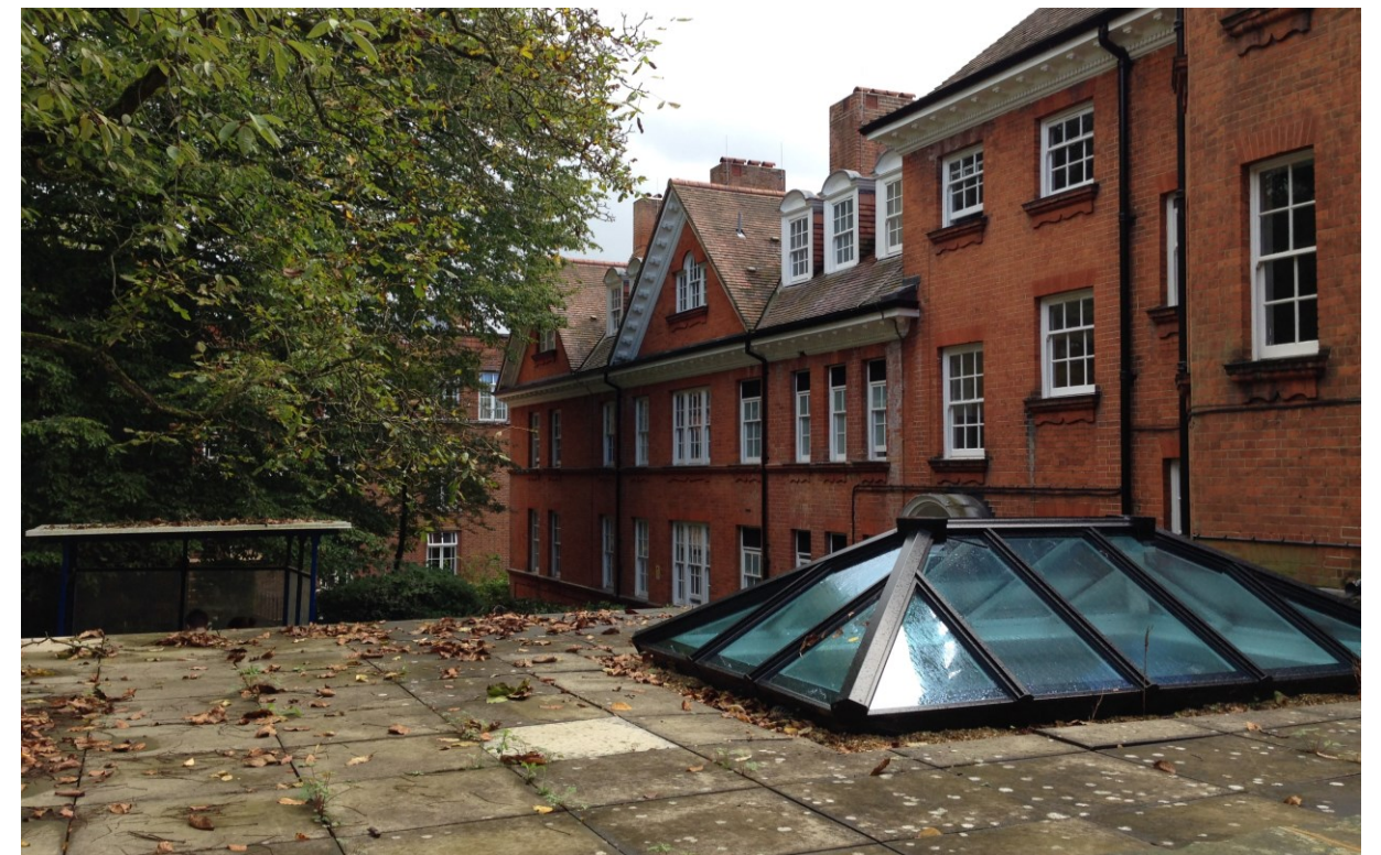
Figure 93. A photograph of the roof of the single storey extension to the rear of Skeel Library and the protruding rooflight.
