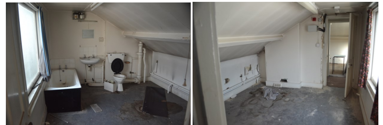
Figure 65. A photograph of a typical bathroom (left) and former bedroom (right) at the second floor level.
