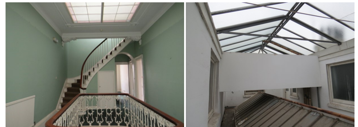
Figure 66. A photograph of the decorative skylight seen from a location on the first floor level landing, and the second floor level, and the structure located over the skylight at the second floor level.
