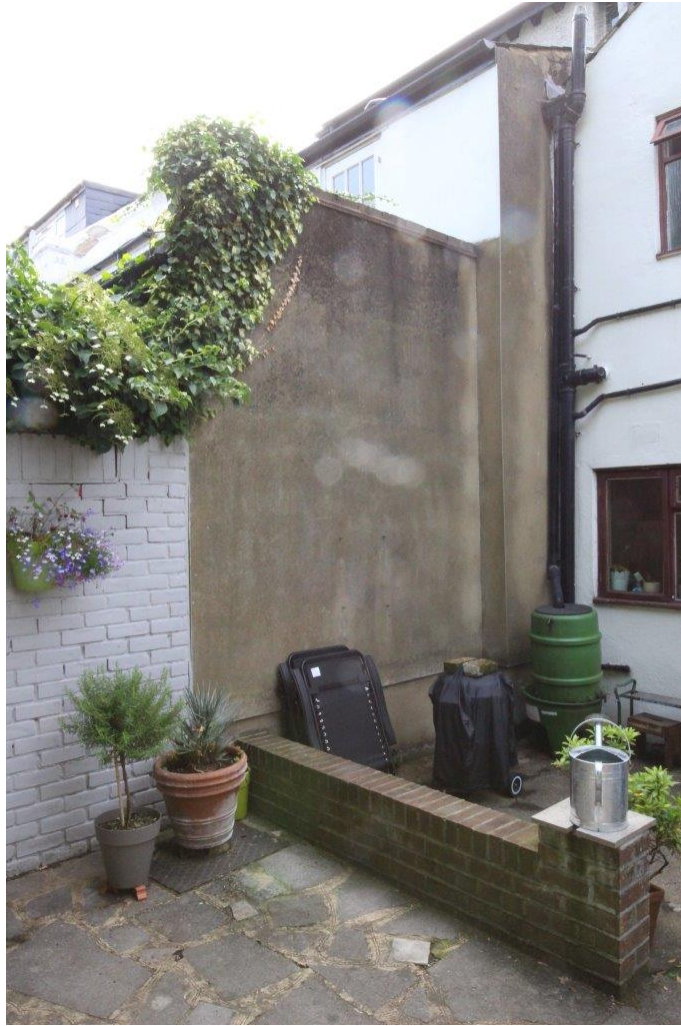
3. View of the rear elevation showing the relationship between No. 8 and No. 7 to the LHS – a flank wall
