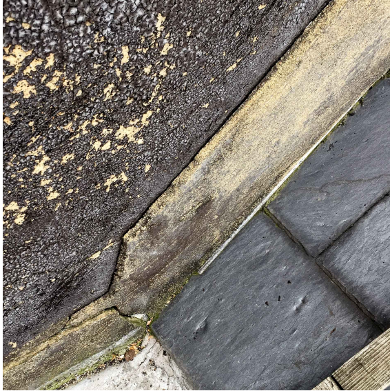
Image 8, View Cement Render to Chimney Breast.
