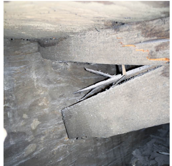
Image 6, View of Failed Blocking Member Within First Floor.
