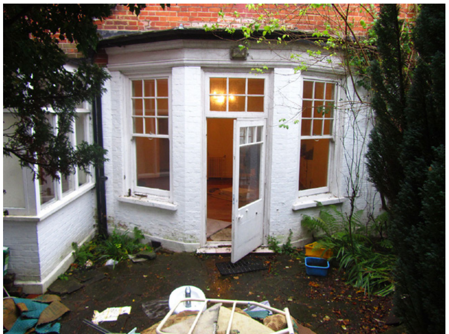
The rear elevation, as existing, showing the original bay and 'link' extension (to the left).
