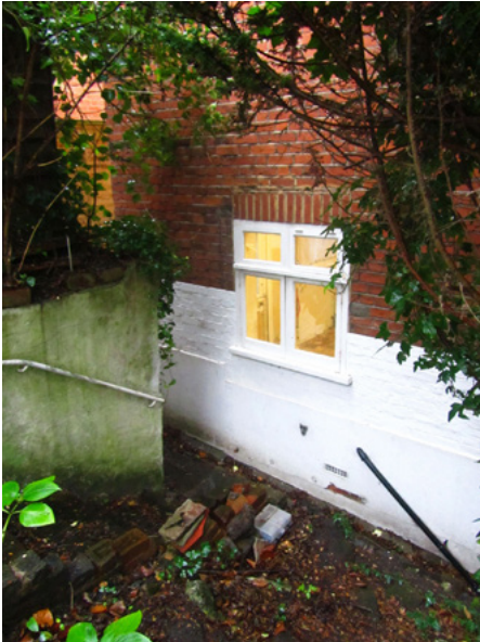
Existing rear elevation, showing the kitchen window set within the closet wing.
