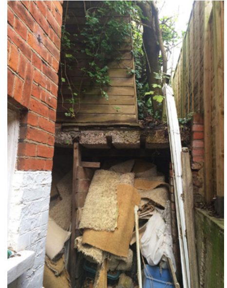
Existing unsafe coal bunker and other associated structures.
