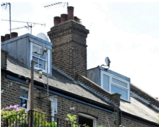
3 Other metal clad dormers to properties to the west on Mansfield Street
