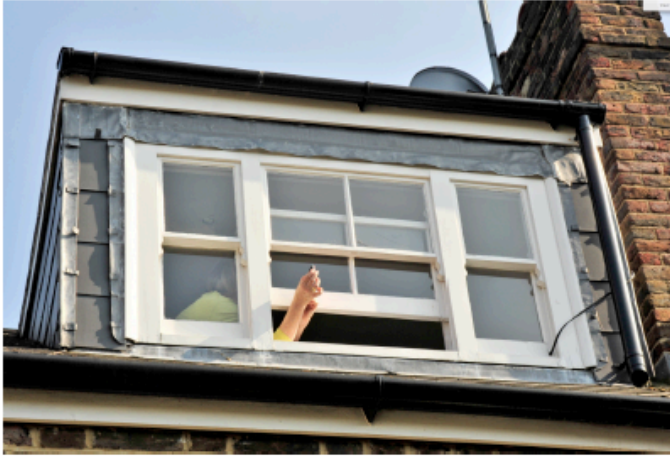
1 Existing dormer at 28 Mansfield Road, showing slate and clumpy lead detailing
