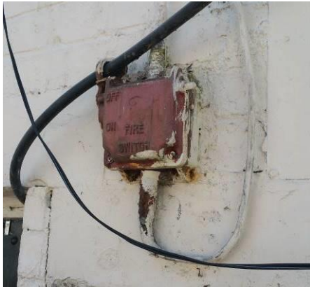
Suspected isolator switch
