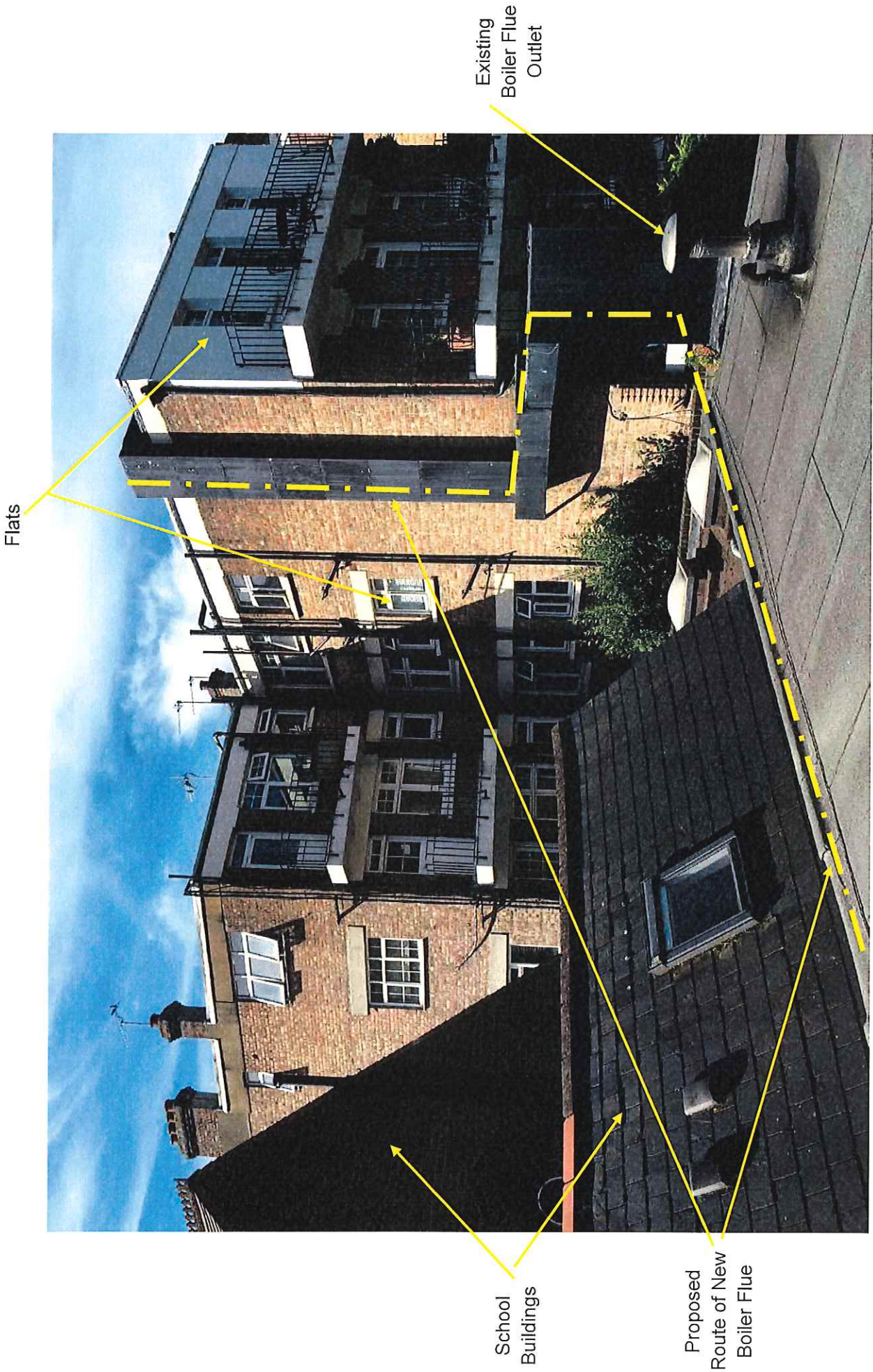
Photo C – Location of Existing Boiler Flue at Other End of Boiler House Roof
