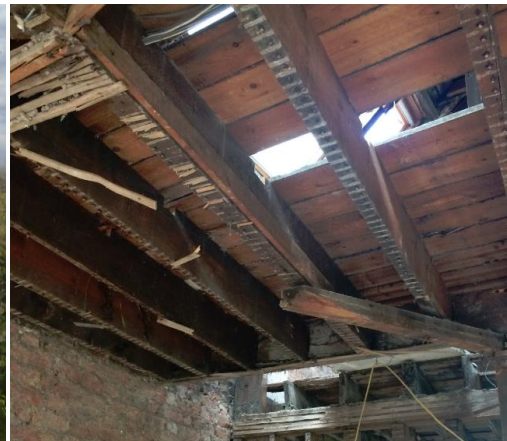
POOR STRUCTURAL FLOOR MAKEUP
