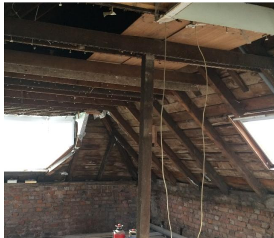
EXISTING ROOF AND FLOOR STRUCTURE IN VERY POOR CONDITION
