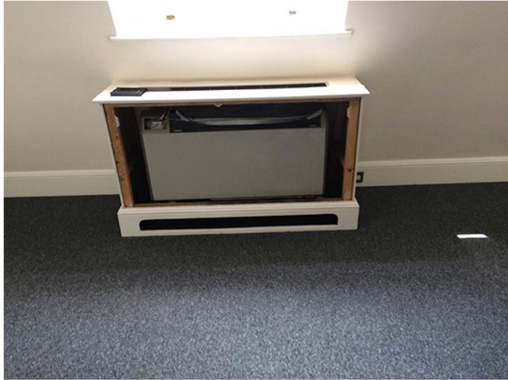
01 - Photo of existing timber boxes laid to conceal / househeating system (Panel removed)
