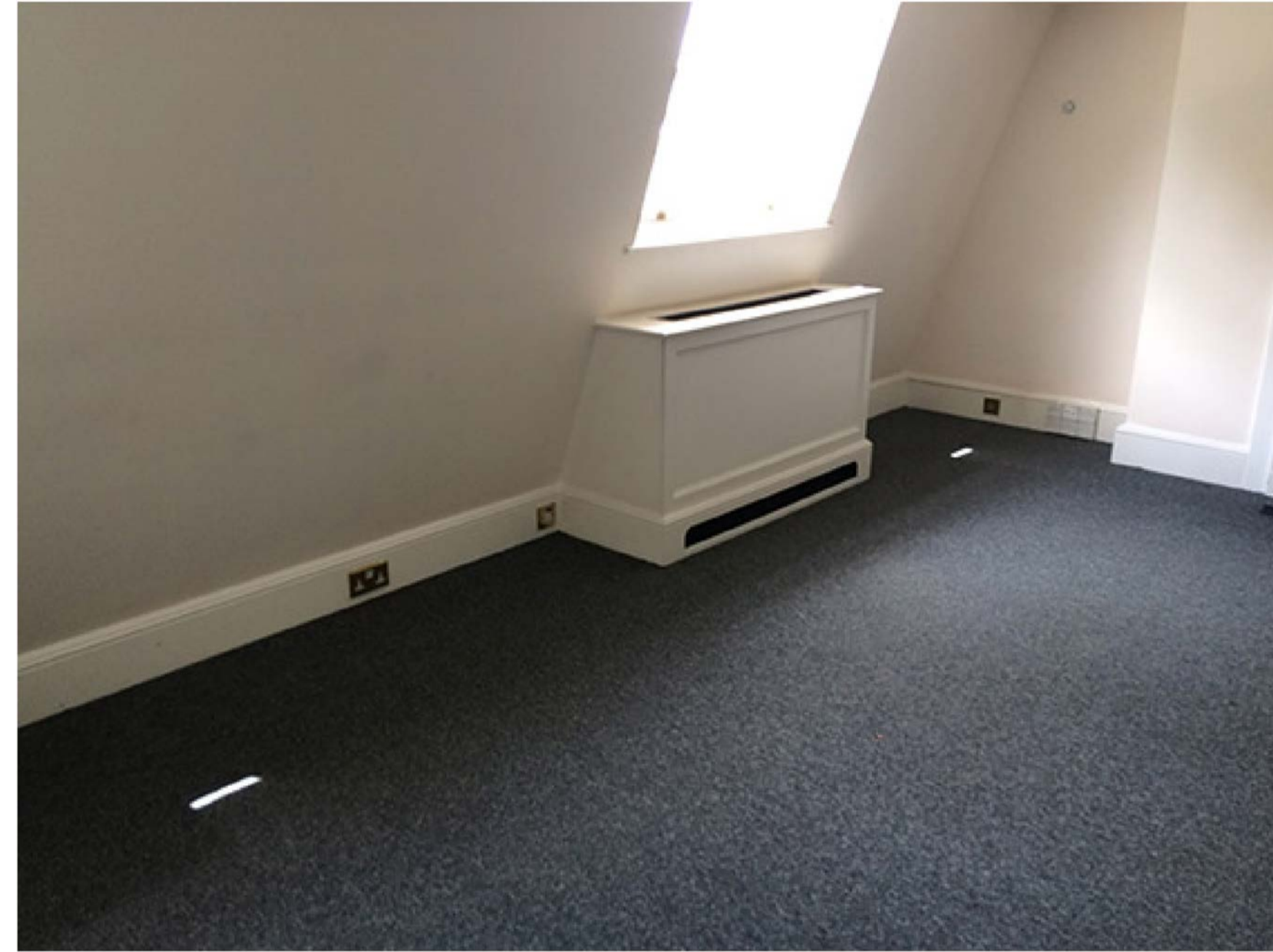
02 - Photo of existing timber boxes laid to conceal / househeating system
