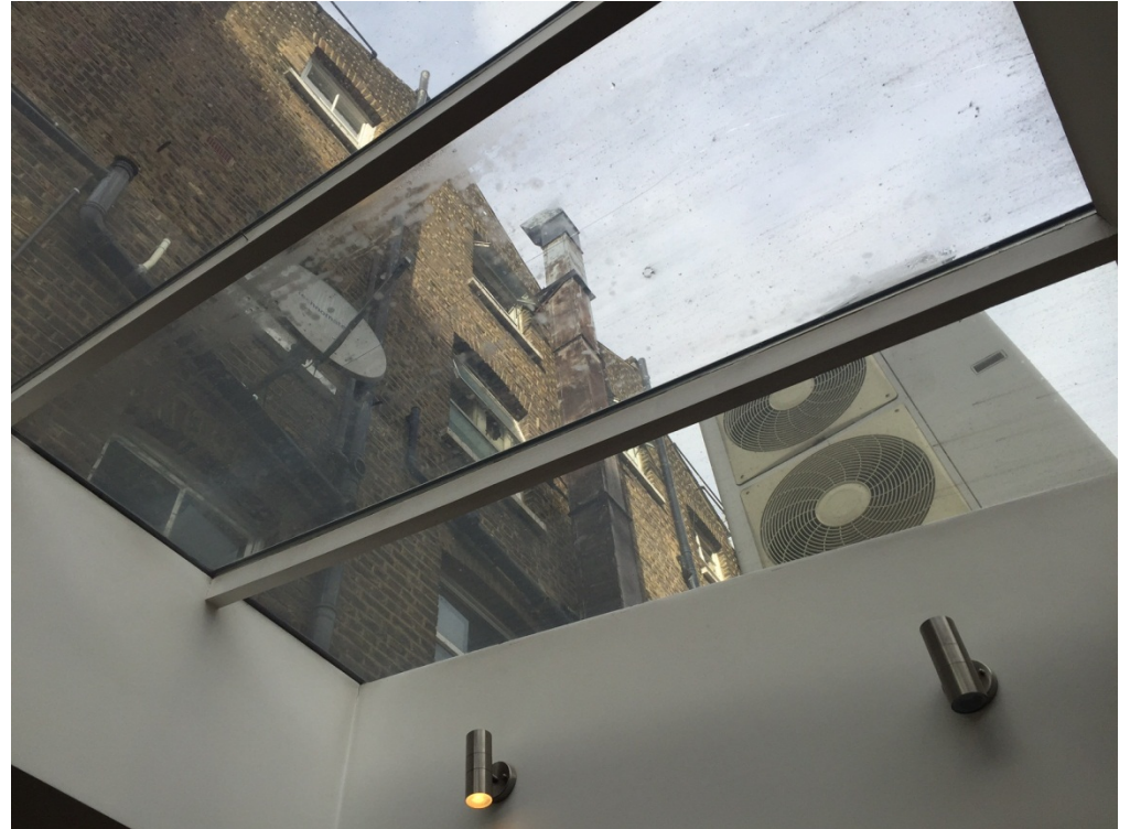
View of rear elevation to existing air conditioning units at 35 Theobald's Road
