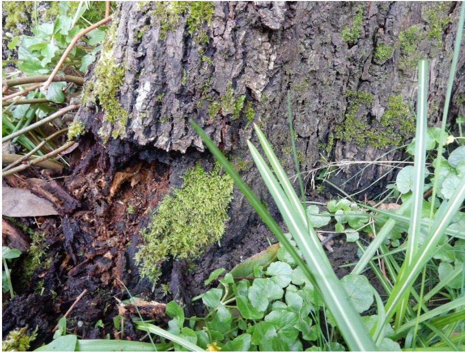
Photograph 3. Decayed buttress at base of Tree 8
