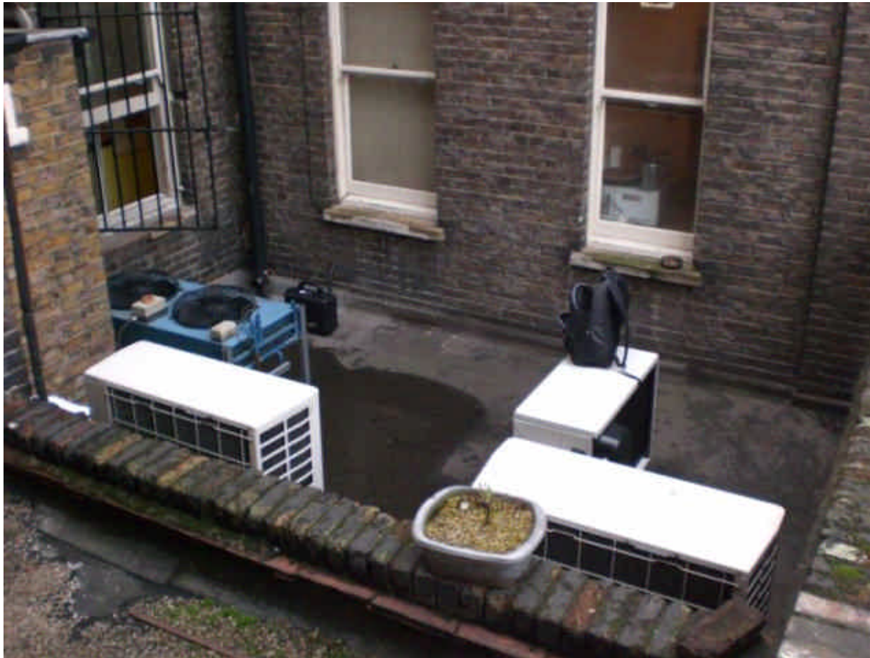
Existing Mechanical Plant on flat roof
