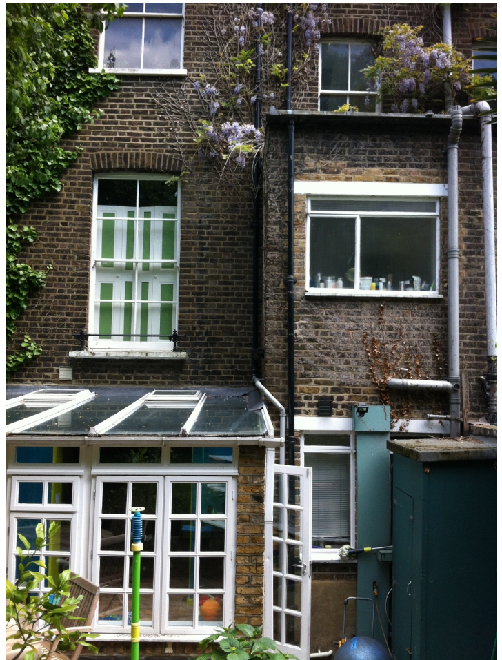
The closet wing with metal-framed windows. The boiler and hotwater tank is housed in a timber enclosure.
