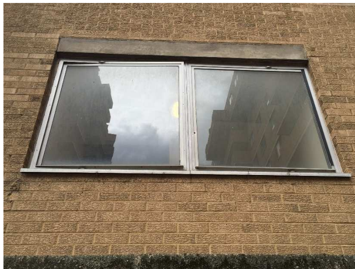
Photograph 1: Existing aluminium vertical pivot window in a communal area at No2 Greville Street
