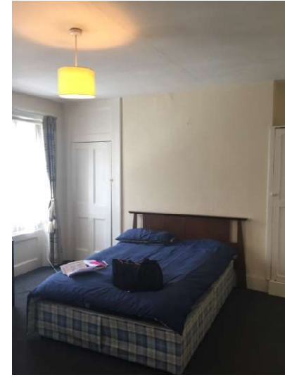
Plate 15. Boxed in chimney breast, no cornice
