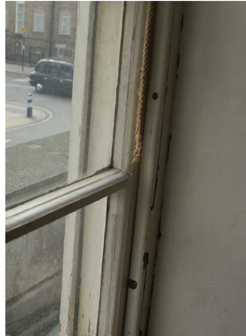
fig. 5 - Broken counter-weight rope.
