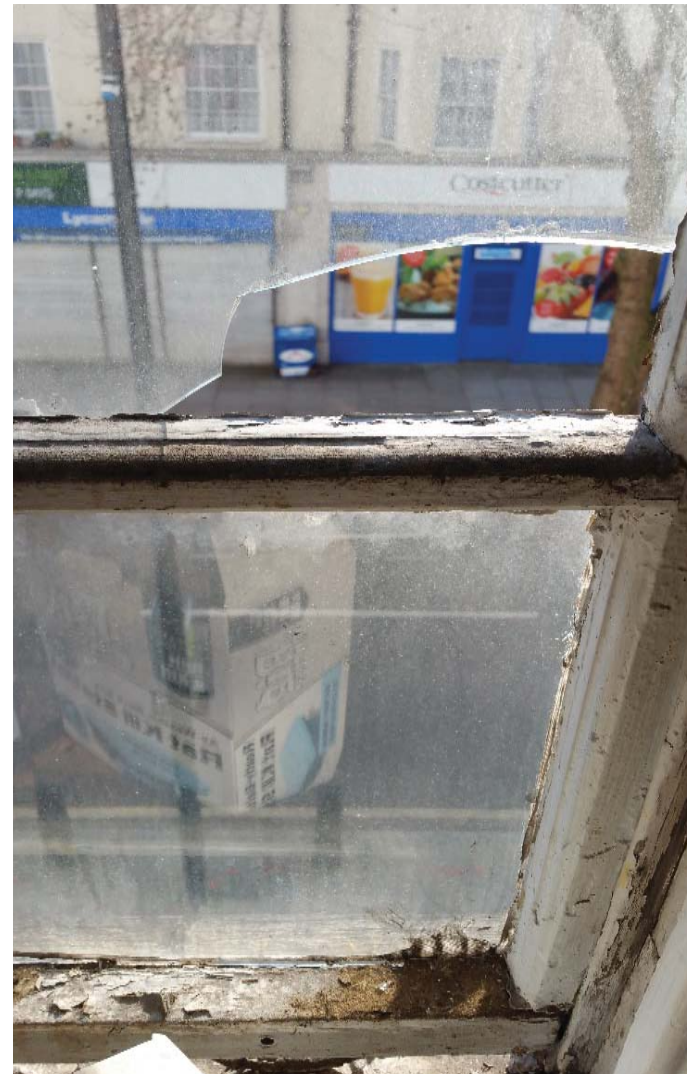
fig. 7 - Broken glass panel on lower sash.
