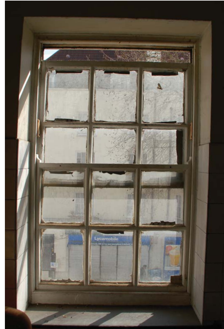
fig. 6 - Sash window interior condition. Damaged glass panels held in frame by old putty.
