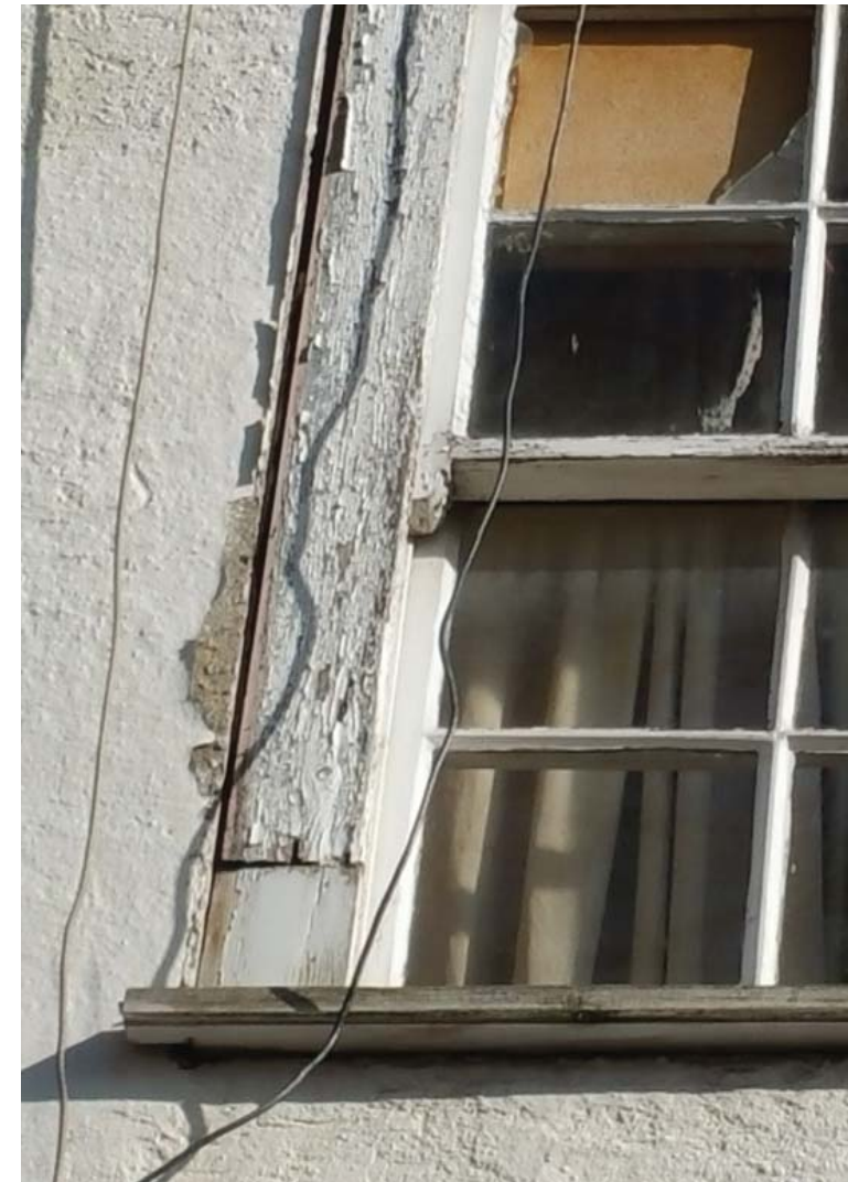
fig. 3 - Shattered glass panel. Damaged frame, coming away from brickwork.
