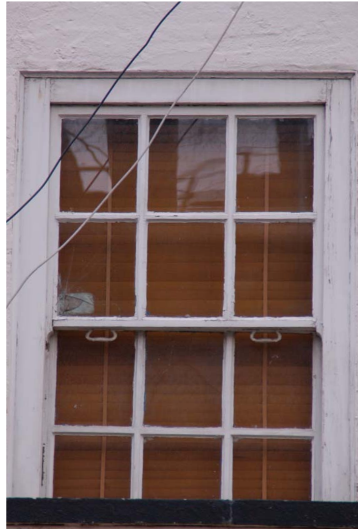
W1 02 Rotten cill, beyond repair. Damaged runners and window lock. External sash handles need re-fitting. Bottom rail to top sash rotten. External box severely damaged beyond repair. Glazed window light broken.
