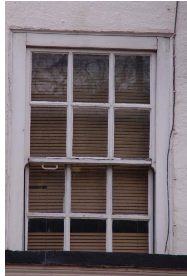
W1 03 Rotten cill, beyond repair. Bottom rail to top sash rotten. Damaged runners and window lock. External sash handles need re-fitting. External box severely damaged beyond repair.
