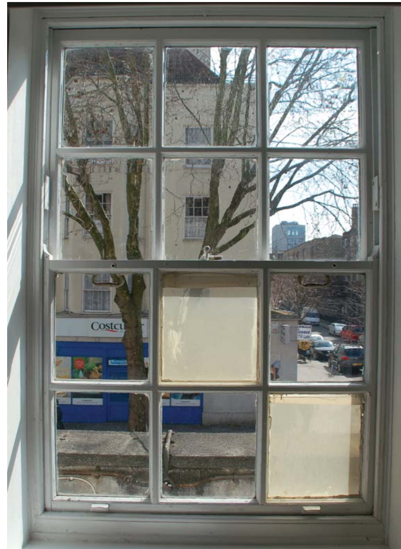
fig. 4 - Mismatching glass panels.
