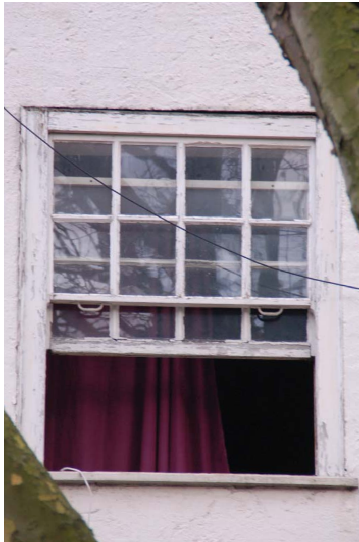
W2 01 Rotten cill, beyond repair. Damaged runners and window lock, replacements required. Bottom rail to bottom sash rotten. External sash handles need re-fitting. External box severely damaged beyond repair.
