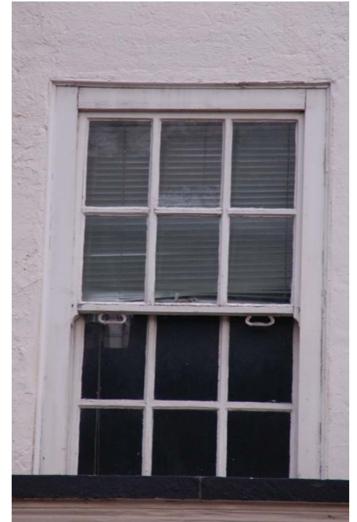
W1 04 Rotten cill, beyond repair. Damaged runners. Bottom rail to bottom sash rotten. Rope for pulley damaged and window requires re-weighting (see fig. 1). External sash handles need re-fitting. External box severely damaged beyond repair.
