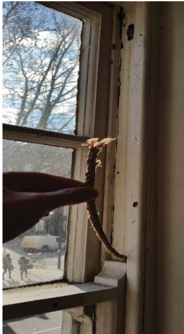
fig. 1 - Rope for window's counter weight system torn.
