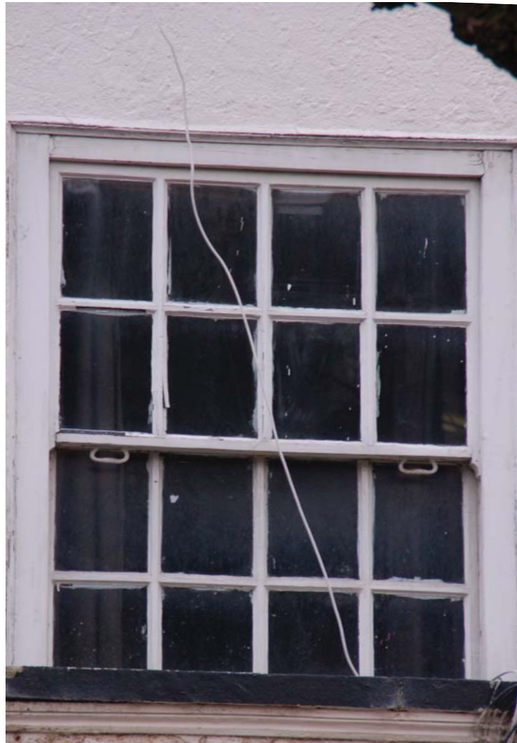
W1 01 Rotten cill, beyond repair. Damaged runners and window lock. External sash handles need re-fitting. External box severely damaged beyond repair. Glazed window light broken.
