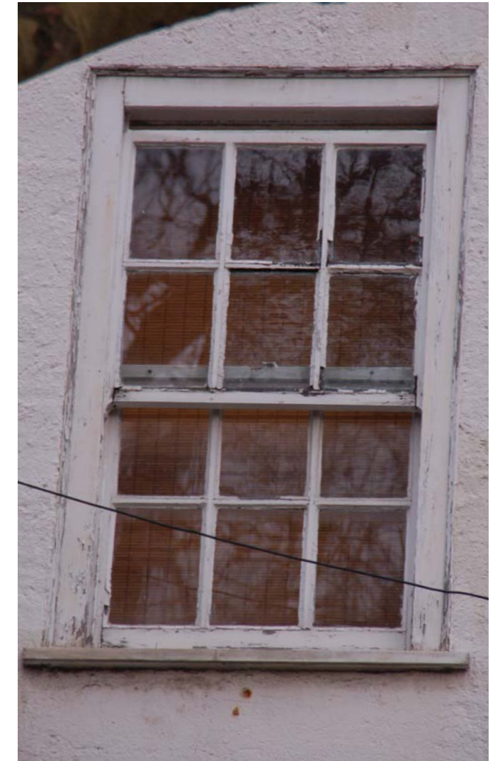
W2 04 Rotten cill, beyond repair. Damaged runners and window lock. External box severely damaged beyond repair.
