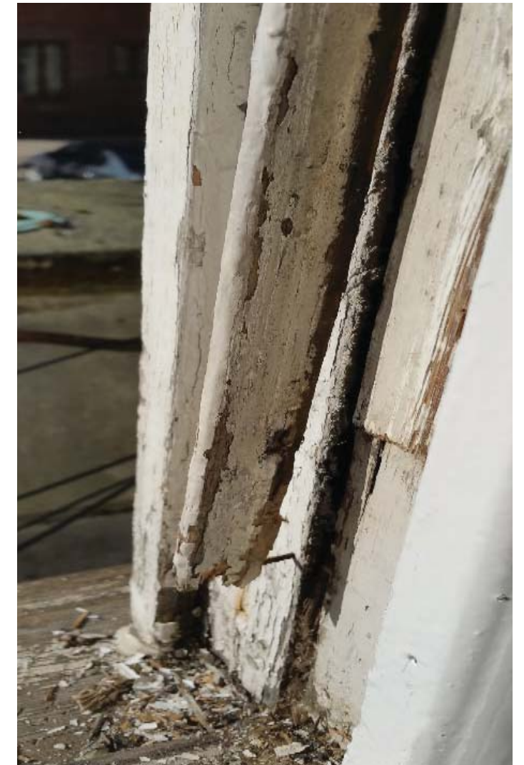
fig. 2 - Rotten box, runner and cill which are beyond repair
