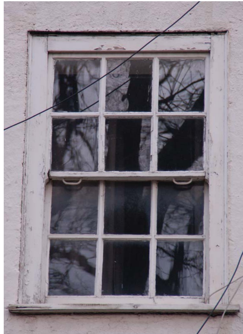
W2 02 Rotten cill, beyond repair. Damaged runners and window lock. External sash handles need re-fitting. External box severely damaged beyond repair.
