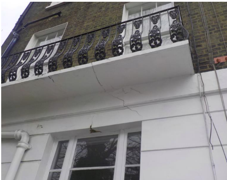
Ground floor window and 1 st floor balcony (balcony belonging to 88a Albert Street, neighbour)
