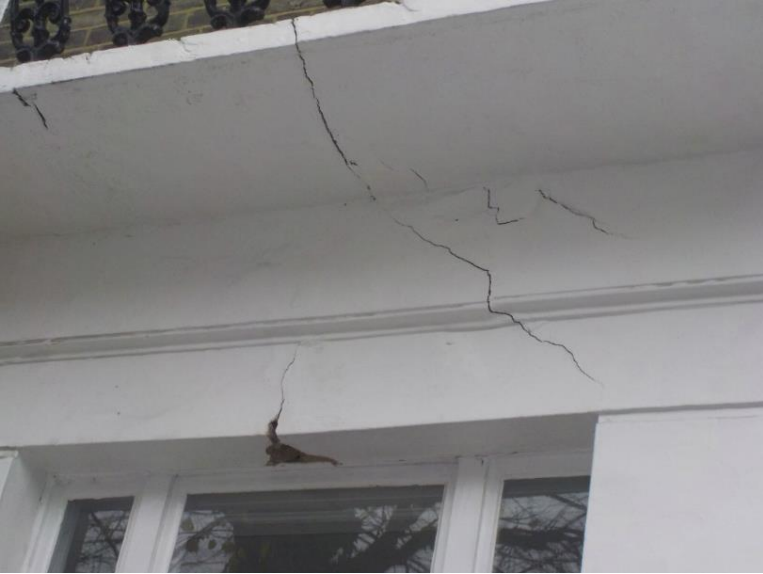
Ground floor window and 1 st floor balcony (balcony belonging to 88a Albert Street, neighbour)
