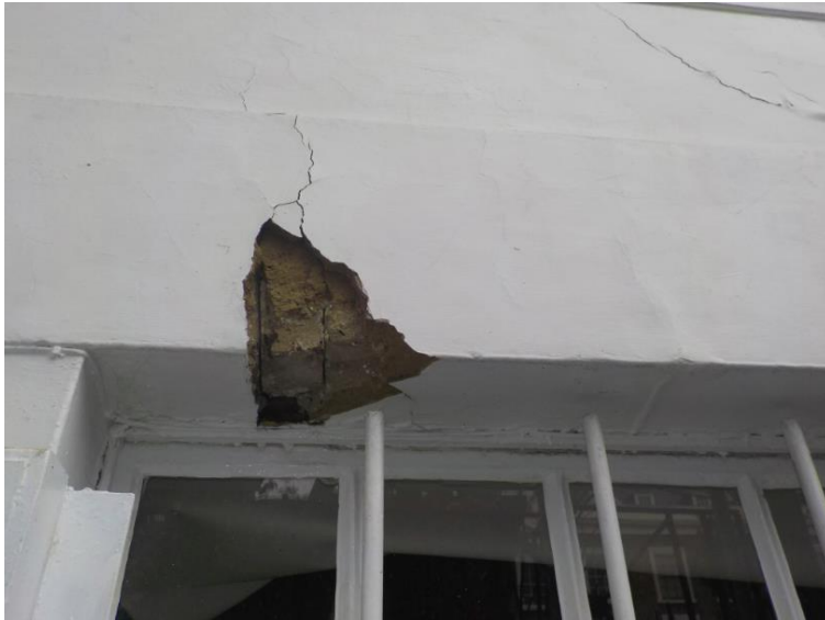
Lower ground floor window, partial rendering removed to expose that the concrete lintel is broken
