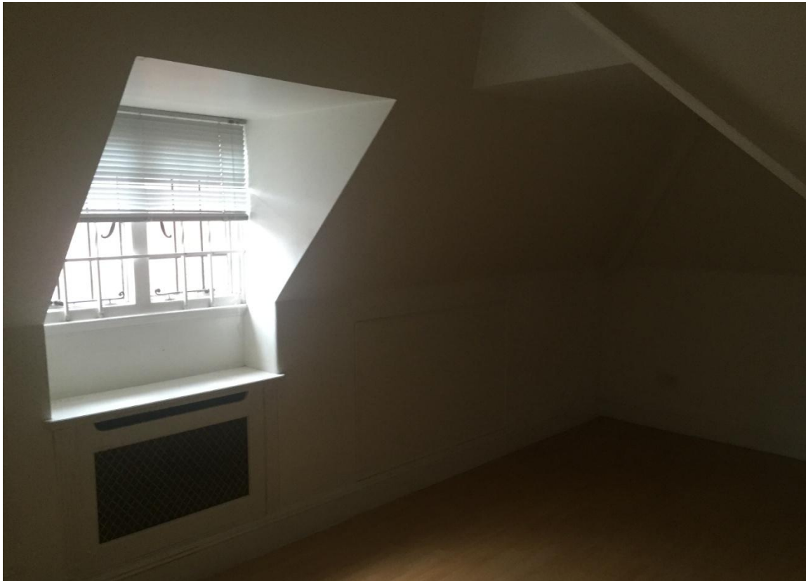
Figure 3 - Accommodation on the existing second floor level is limited in terms of usable head height
