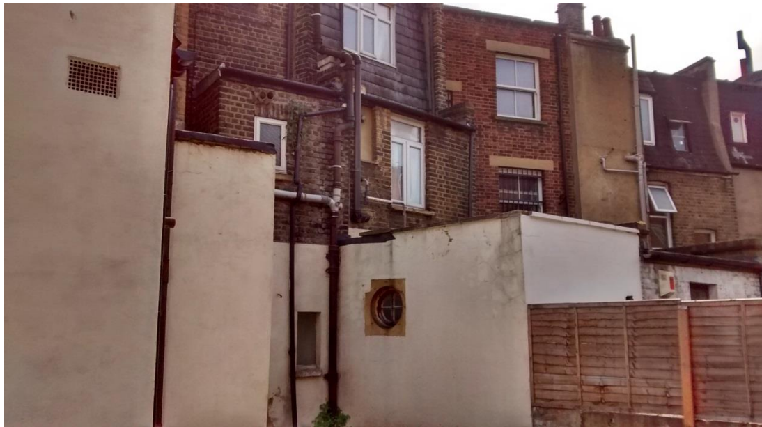
Existing rear elevation of 111 Kentish Town Road including single storey half width rear extension, with view towards existing rear extension at 109 Kentish Town Road
