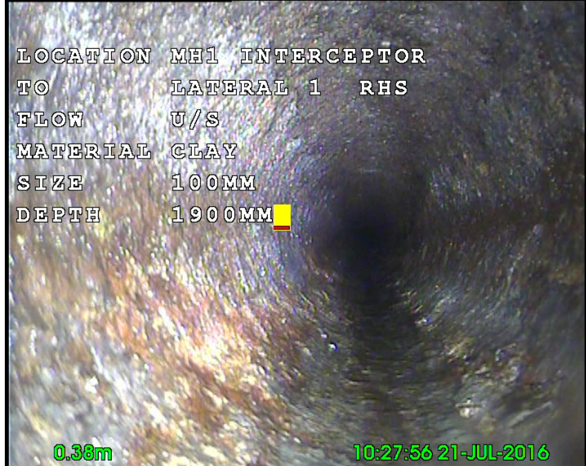
Photo: 3_4_20_A.jpg 0.3m, Attached deposits, encrustation, from 12 to 12 o'clock, 5% cross-sectional area loss, Start
