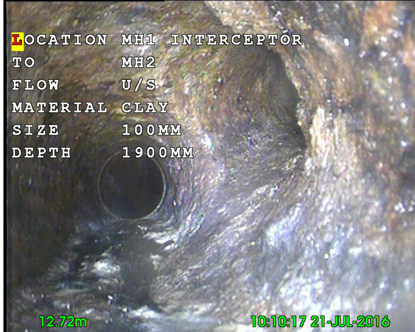
Photo: 1_1_5_A.jpg 12.72m, Junction, at 3 o'clock, diameter 100mm
