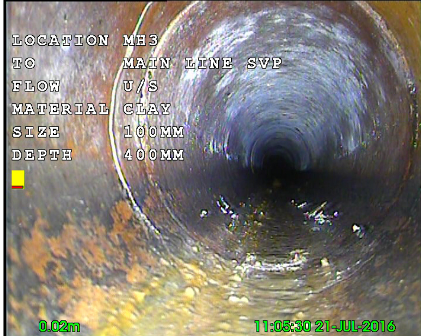
Photo: 5_6_32_A.jpg 0.02m, Fracture, circumferential, from 6 to 12 o'clock
