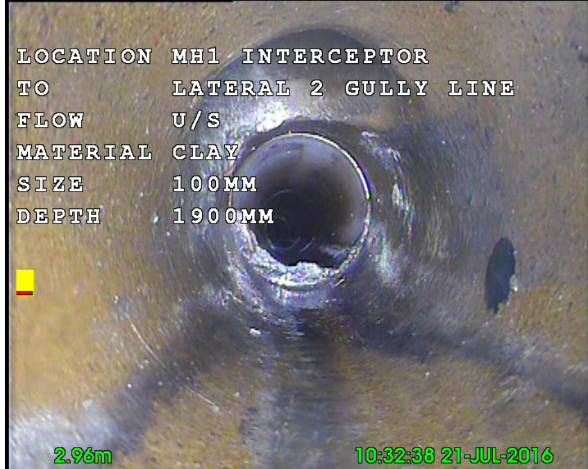
Photo: 4_5_26_A.jpg 2.96m, Junction, at 12 o'clock, diameter 100mm
