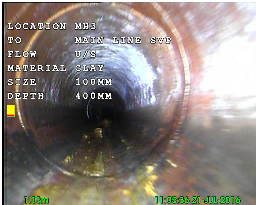
Photo: 5_6_33_A.jpg 1.11m, Fracture, circumferential, from 12 to 12 o'clock
