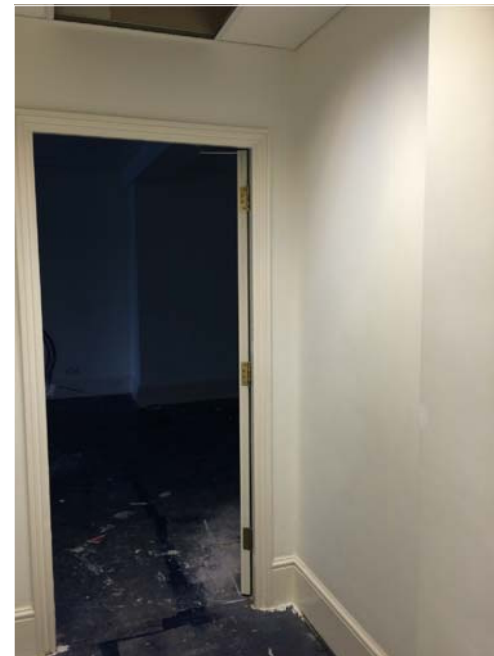
Photo 6 SECOND FLOOR: OPENING to BE CREATED in NON-ORIGINAL STUD PARTITION & SINGLE DOOR to BE FITTED
