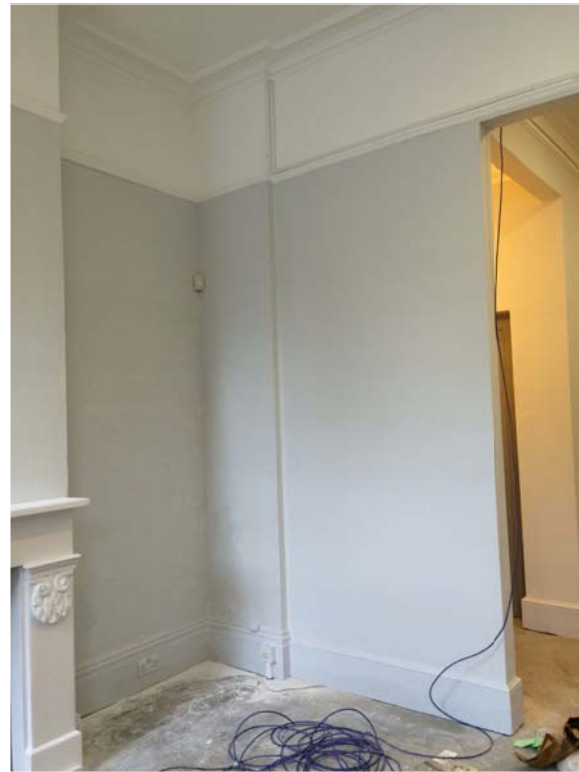
Photo 2 GROUND FLOOR: NON-ORIGINAL STUD PARTITION to BE REMOVED
