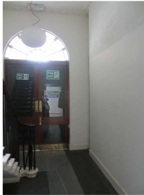
Photo 3 GROUND FLOOR: ORIGINAL OPENING to BE REINSTATED & DOUBLE DOOR FITTED
