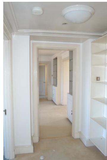
View through the breach in the party wall from the north into the south house
