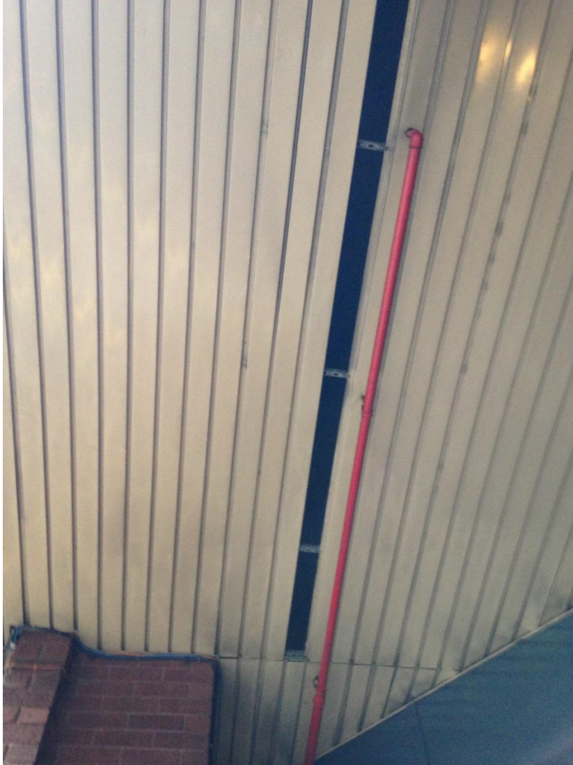
Plate 3: Missing aluminium panel above basement vehicle entrance.
