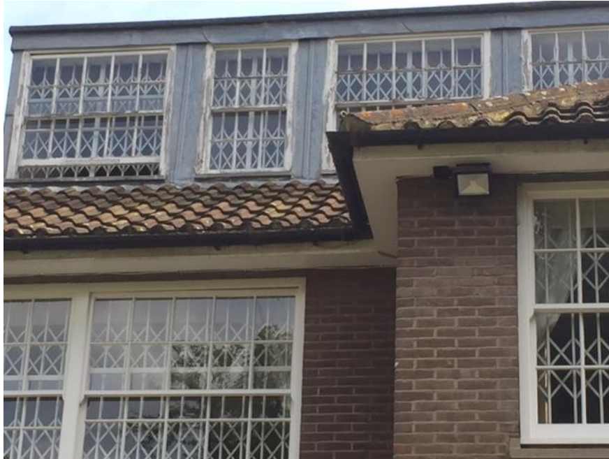
Figure 4.3 View from ground of one of the pitched sections of roof showing small number of gaps under lead flashing and hanging clay tiles.
