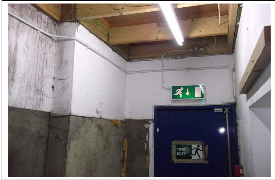
The above picture shows the right hand fire exit corridor with plastered brick work walls, a painted concrete floor and metal fire exit door, wooden roof materials and joists and a wooden door to the workshop.
