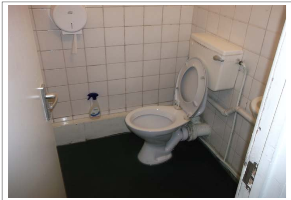
The above picture shows the toilets with plastic and ceramic sanitary ware, cast iron and plastic pipe work and wooden boxing, ceramic wall tiles and a plastered ceiling.
