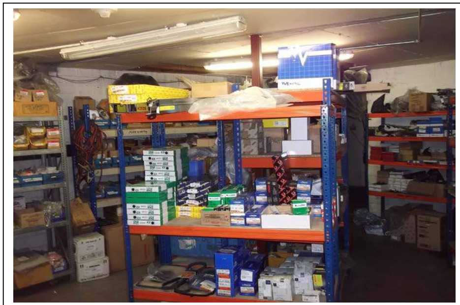
The above picture shows the commercial store room with a painted concrete floor, brick work walls and a plasterboard ceiling below wooden joists and chipboard decking of the above mezzanine floor, there is a plastic downpipe and wooden door.
