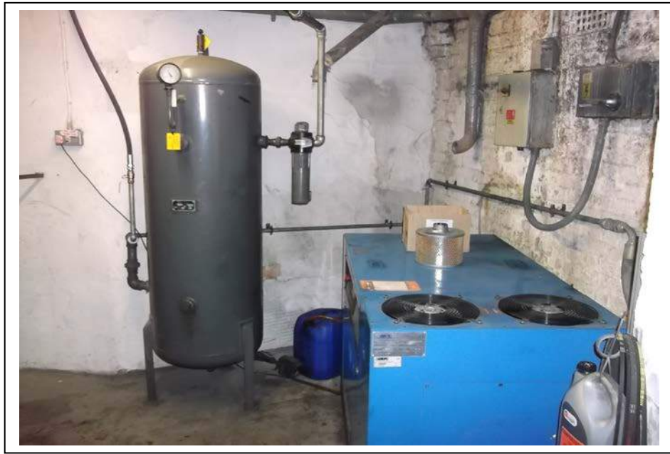
The above picture shows the compressor room with brick work and rendered walls, a concrete floor and concrete ceiling, a modern compressor and air reservoir, modern electrics and ducting, a metal ladder to a wooden door and the roof access.
