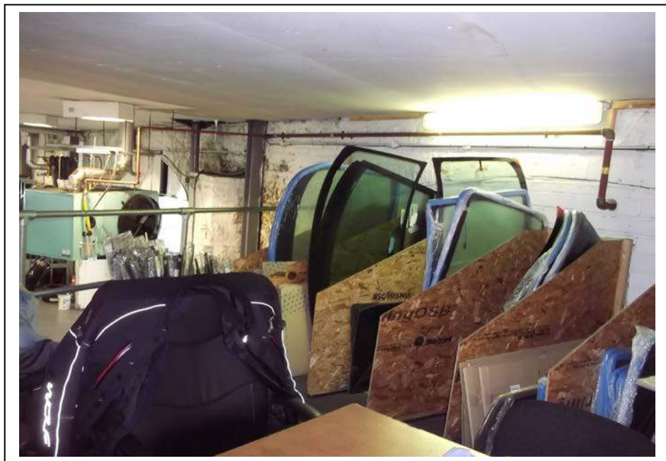
The above picture shows the mezzanine glass store and rest area with wooden decking and metal safety rails, plasterboard ceiling panels below concrete, brick work and wooden materials and RSJ's, there are painted brick work walls and a wooden staircase.
