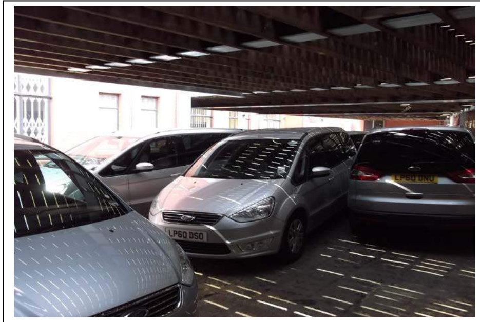
The above picture shows the vehicular store with a concrete floor, painted brick work walls and metal roller door, RSJ's and a wooden roof.
