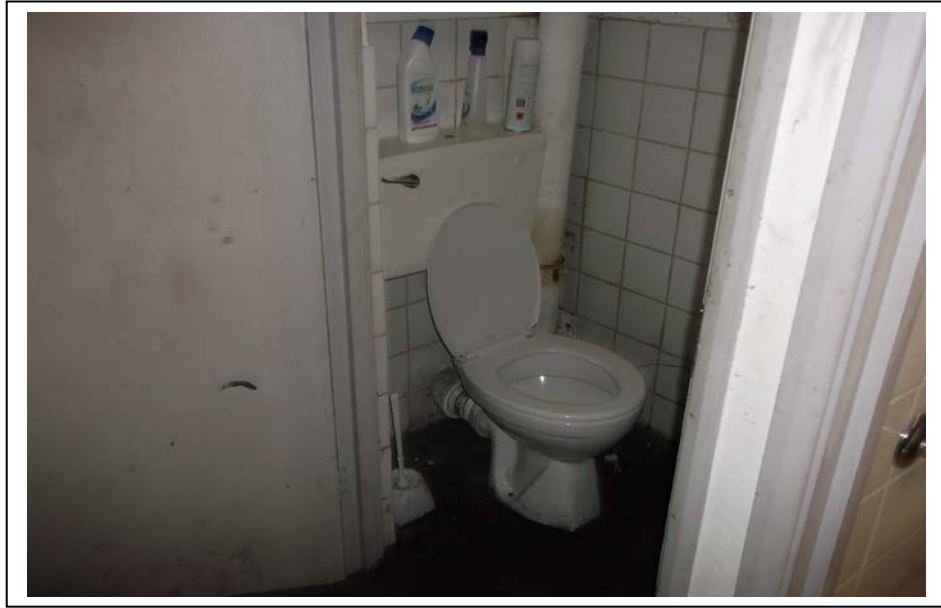
The above picture shows the toilet off the parts store with plastic and ceramic sanitary ware, a wooden doors and concrete floor, ceramic tiled and rendered block work walls.
