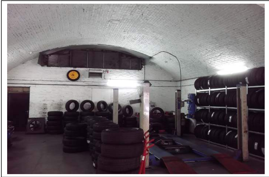
The above picture shows the tyre bay with painted brick work walls and arched ceiling, a painted concrete floor and metal vents to the upper walls, cast iron pipe work and wooden door. This is typical of all areas under the railway arches.
