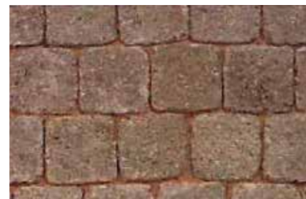
ST1: Permeable Paving
