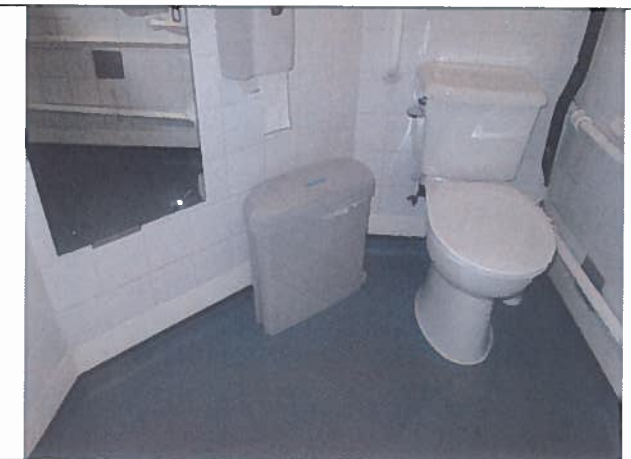
Photo 15: Existing room 220 floor, solid timber door, tiled walls, vinyl floor with covered upstands and Part M install.
