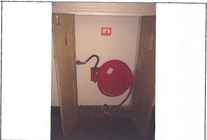
Photo 12: Existing corridor fire hose reel recessed in to Room 125A.
