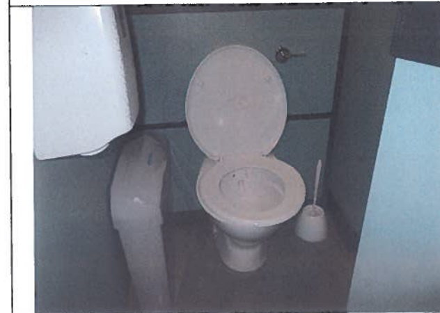
Photo 9: Existing Room 125C pan and concealed cistern behind wall panels.
