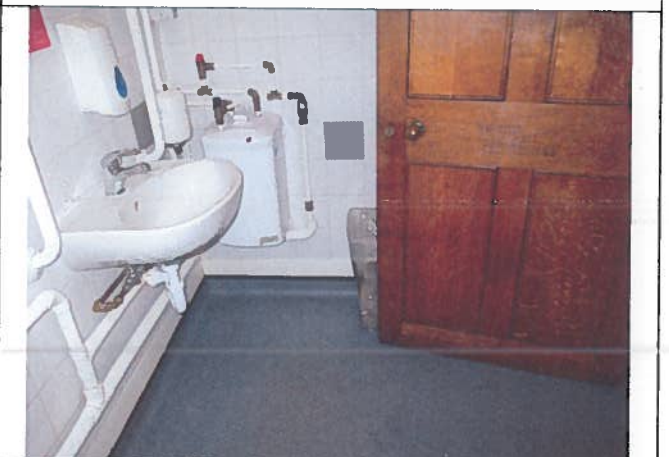
Photo 14: Existing room 220 floor, solid timber door, tiled walls, vinyl floor with covered upstands and Part M install.
