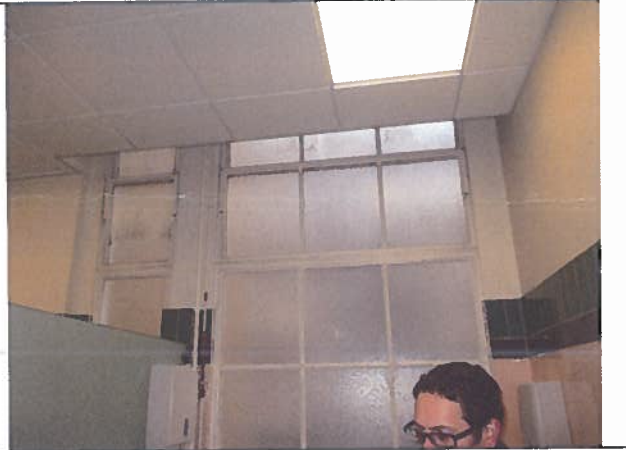
Photo 8: Existing Room 125C metal windows, tiled and decorated walls & suspended ceiling with recessed lights.
