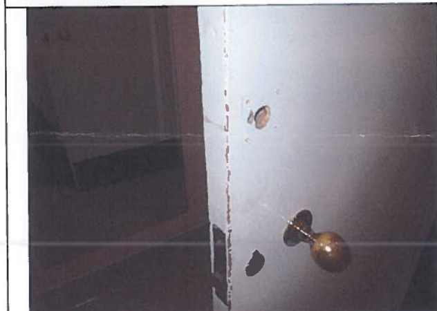
Photo 7: Existing Room 125C solid timber doors to Rooms 125A, 125B and 125C.
