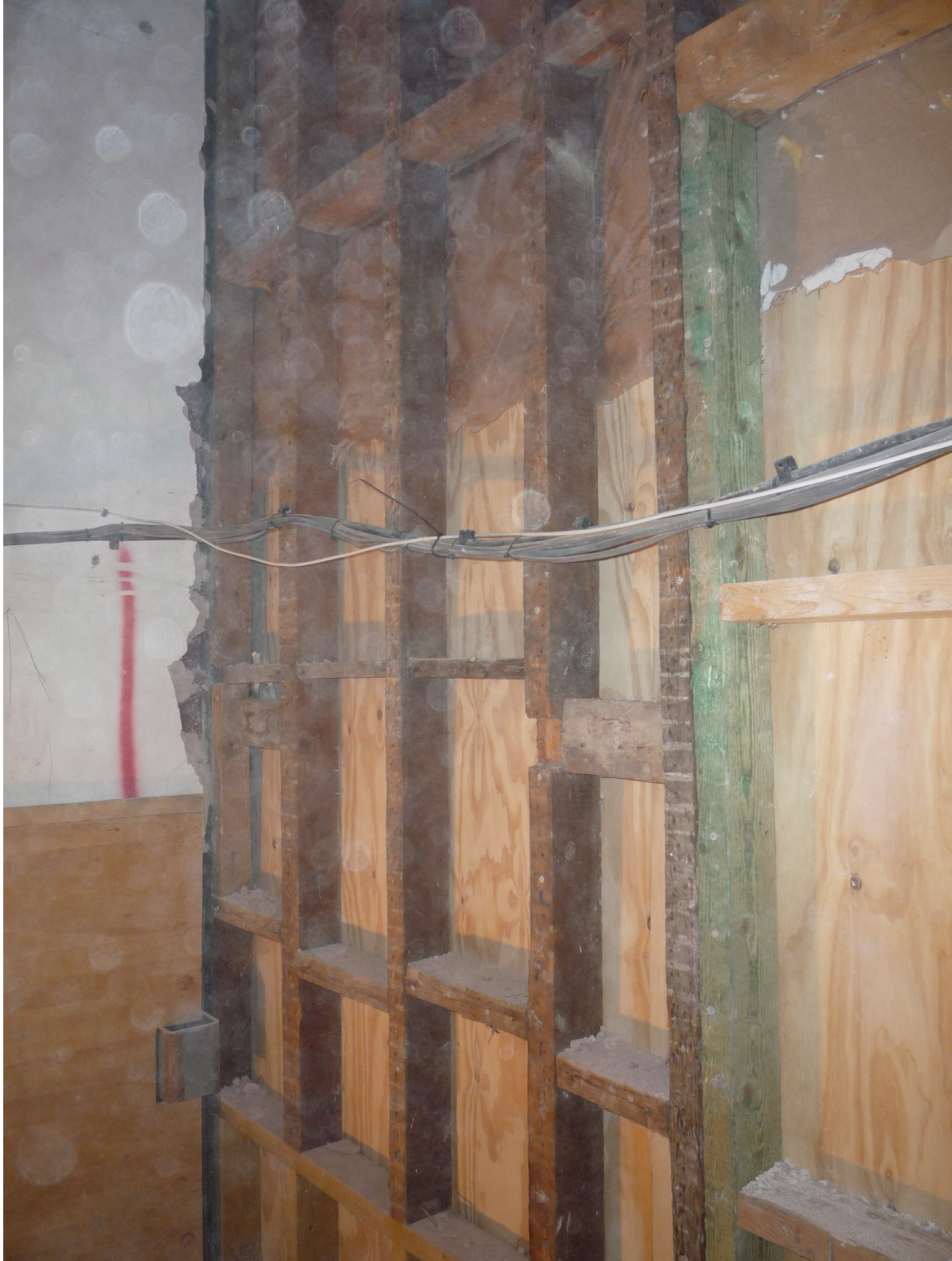
picture taken from the Living Room showing the original / later installed studwork
