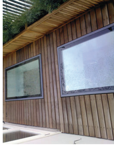
Sample of sky light proposed to be inserted in roof terrace, allowing natural light into the shower room and hall/entrance to new rear bedroom.
