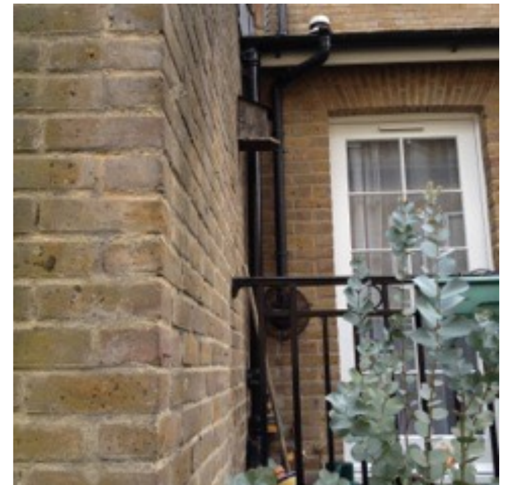
Ground Floor Flue of Neighbouring Property concealed within rainwater pipe
