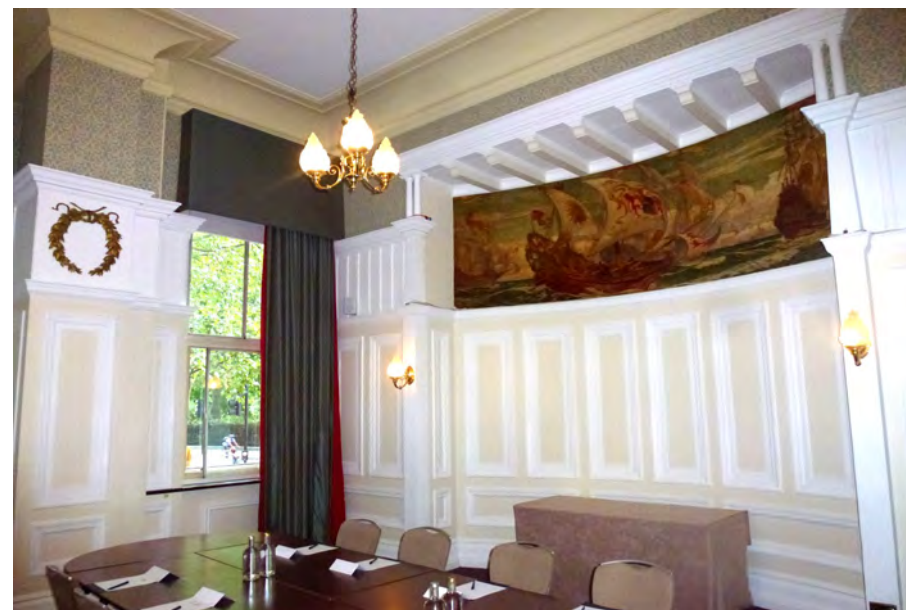
Figure 19: View of the existing King's Bar with the later, curved partition subdividing the space into two. later-applied timber panelling and heavy plaster moulding are present within these rooms. On the north side of the curved partition is a later painting of Tudor-period ships, which bears no resemblance to Doll's original interior.
