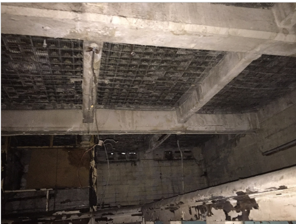
Fig 3. Pavement light underside showing cracking and surface salts.
