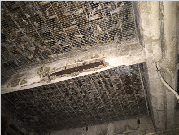
Fig 1. Image beam delamination and spalling, gents side.
