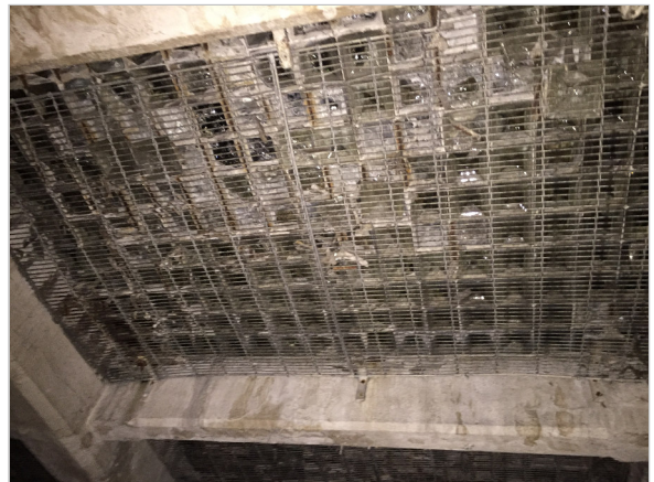
Fig 4. Pavement light underside showing exposed reinforcement and with safety cage installed.
