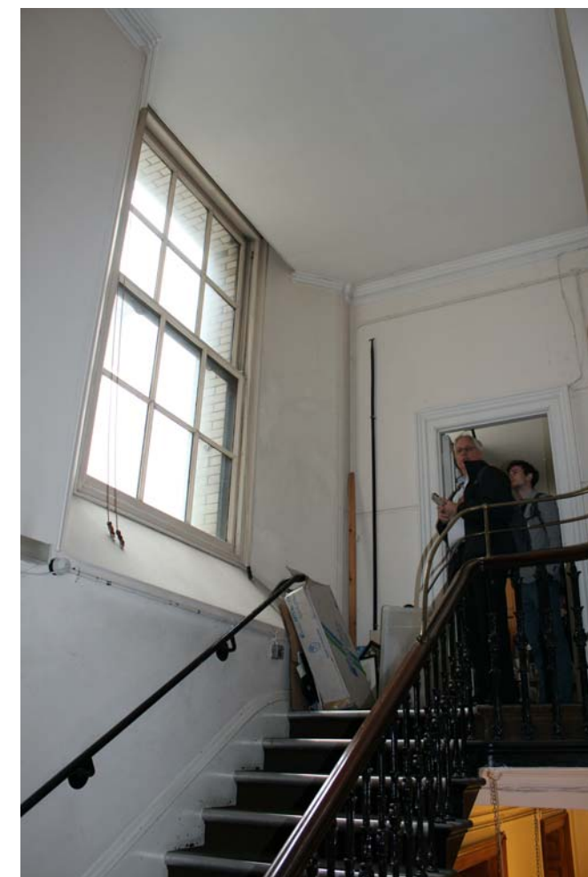
SOUTH SIDE WINDOW ADJACENT EXISTING STAIRCASE TO BE FIRE PROTECTED
