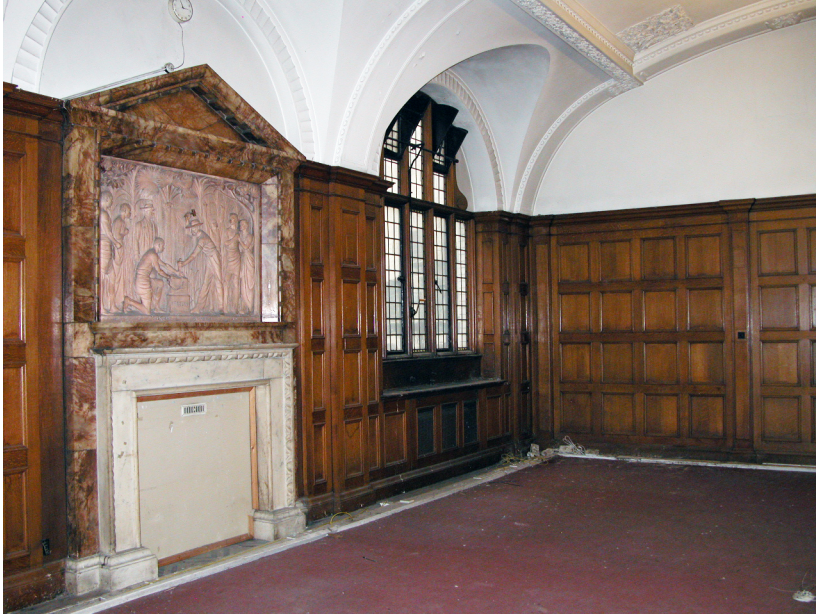
Figure 1: Room 1.05 as existing, showing important features and intrusive trunking for electrical services
