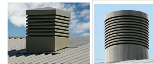
MVHR AND VENT EXTRACT ROOF TERMINATION HEADS APPEARANCE
