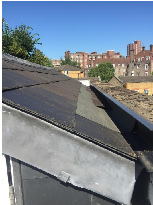
Existing poor quality mansard roof extension.
