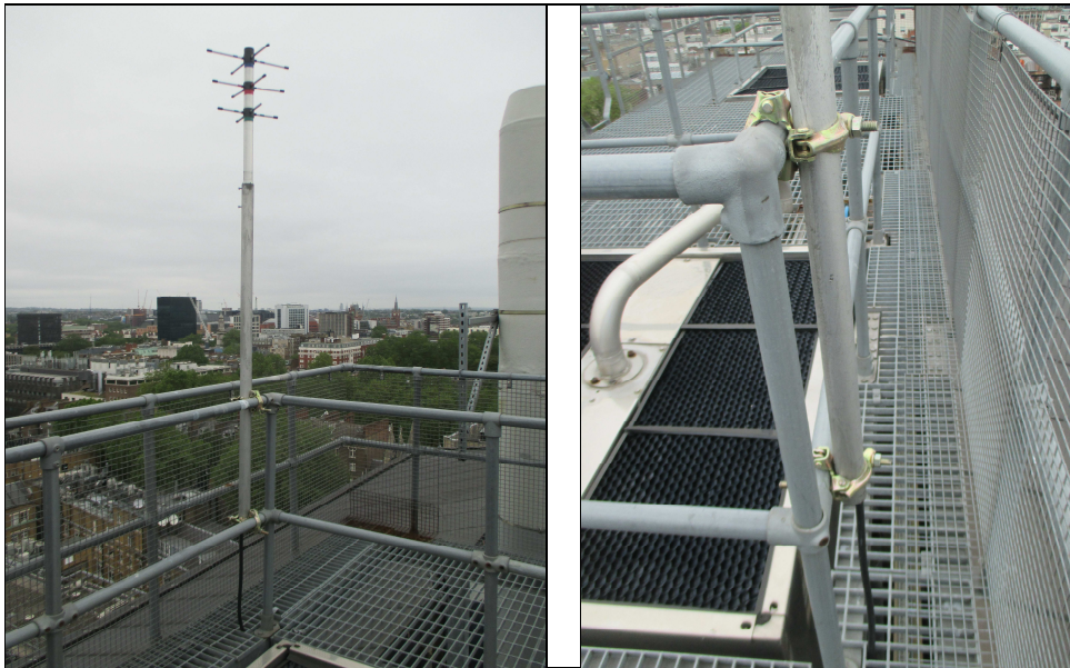
Photo 4 and 5: The existing antenna fixed to the kee klamp handrail of the raised platform floor. The new antenna will match the existing design.
