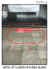
AREA OF SUNKEN PAVING SLABS RAISED PLINTH STONE RAISED 3NO PAVING SLABS
