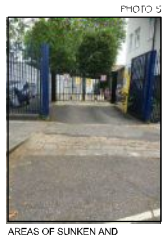
AREAS OF SUNKEN AND CRACKED CONCRETE SECTIONS OF LOOSE CONCRETE AND VEGETATION
