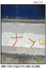
3NO CRACKED PAVING SLABS
