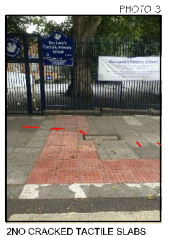
2NO CRACKED TACTILE SLABS 1NO CRACKED PAVING SLAB 2NO CRACKED PAVING SLABS TO SURFACE GULLY
