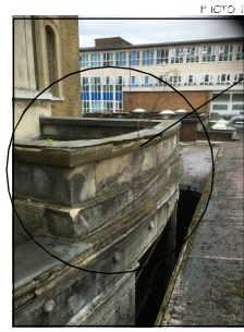
POOR STONE REPAIR LOOSE REPAIR, RISK OF FALLING
