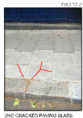
2NO CRACKED PAVING SLABS
