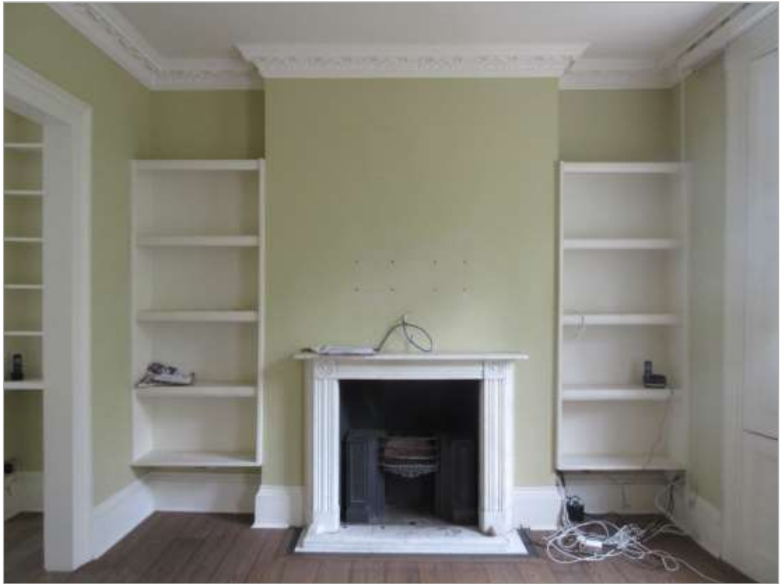
4l: Rear ground floor room, with modern cornices, Regency-style chimneypiece and plastic floorboards
