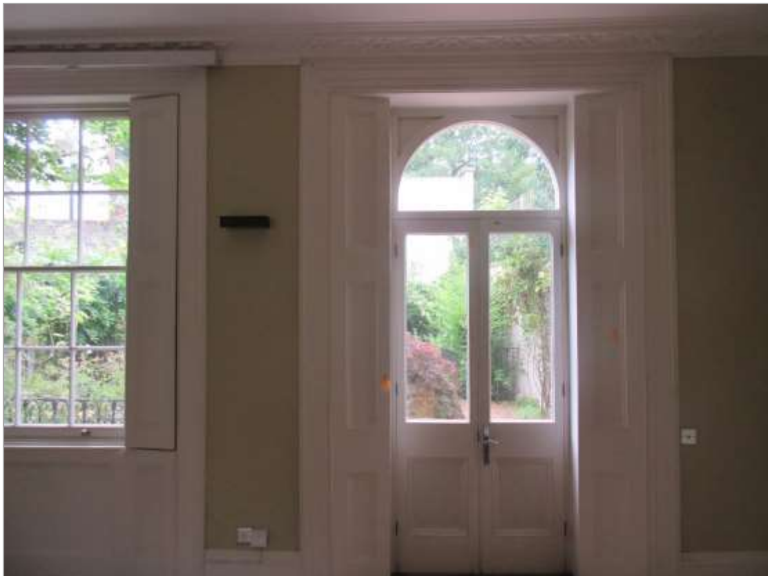
4k: Ground floor rear room, sash window with shutters to left, modern door to right
