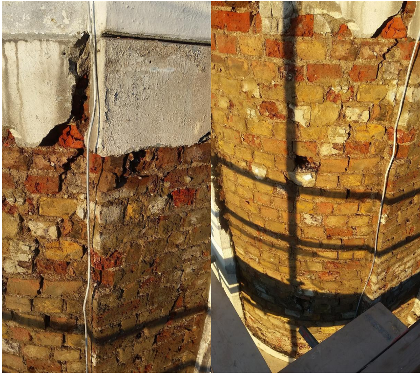
Photo6 – Various cracks present in the existing brickwork.
