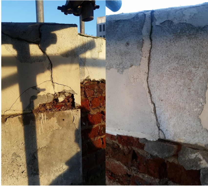
Photo 7 – Various cracks present in the existing render.
