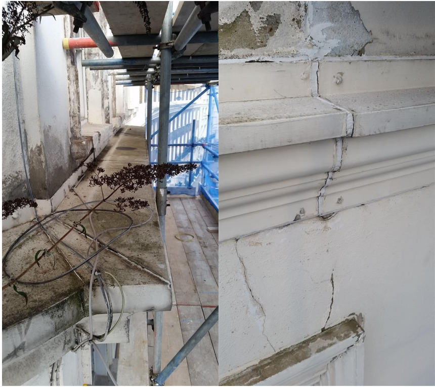
Photo 5 – GRP Mouldings to be reinstated.
