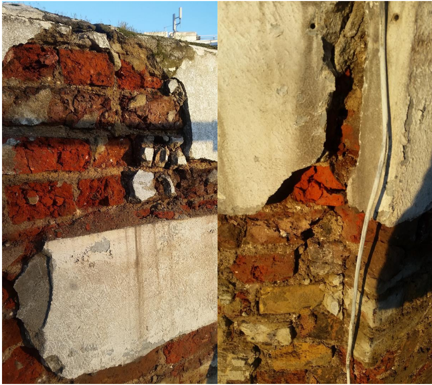
Photo 4 – Defective Brickwork on Front/Flank Elevation
