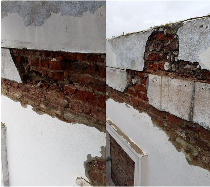
Photo 3 – Brickwork on flank elevation in poor condition
