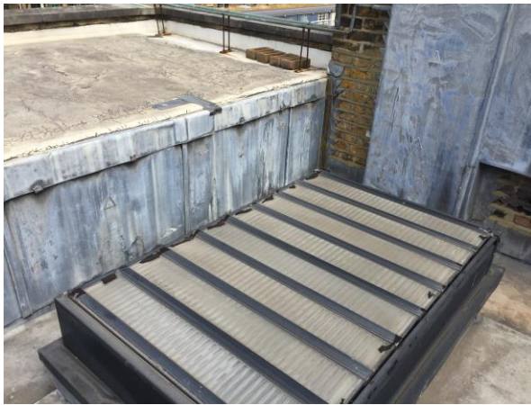
Figure 1: Smoke Vent located on modern addition of 25 Bedford Square
