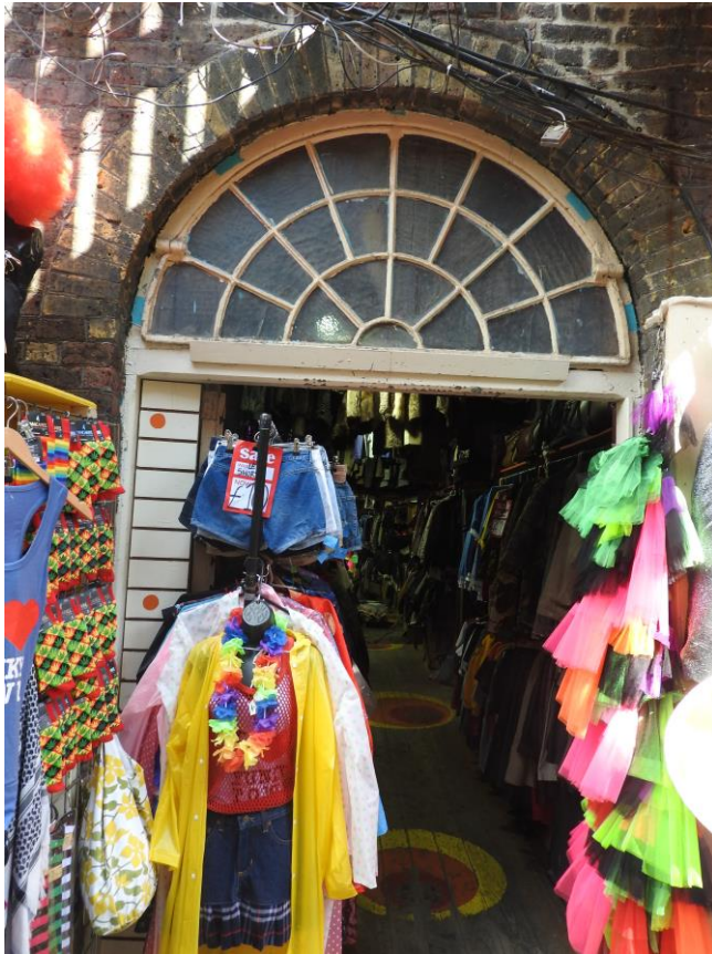
Figure 13 Provender Store west elevation. The original cast iron fanlight will be restored and a new leaf and a half timber door fitted within the repaired historic timber door frame.
