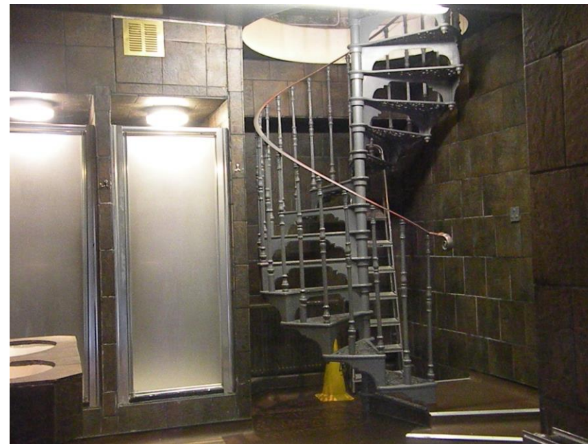
Figure 10 Provender Store first floor showing modern showers and spiral staircase to second floor all to be removed.
