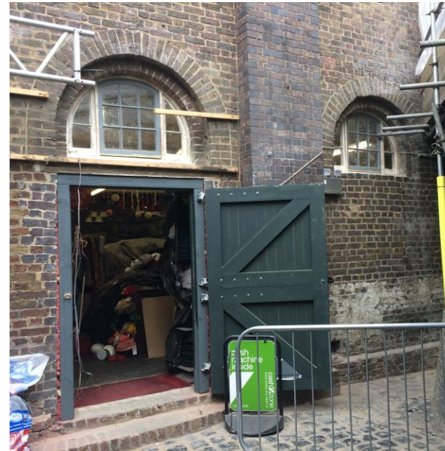
Figure 12 Provender Store east elevation. A new door is proposed below the right hand window which will provide access into the new internal circulation core.
