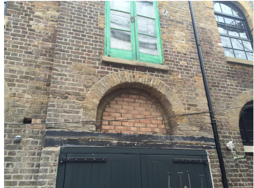
Figure 14 Provender Store north elevation. The brick infill is to be carefully removed from the blocked window aperture and the lunette type window reintroduced.
