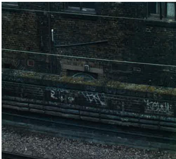
Figure 15 Provender Store south elevation viewed from across the railway. The modern concrete lintel over the door at first floor level will be carefully removed and the curved brick arch lintel reinstated to match that to the west end of the south elevation.
