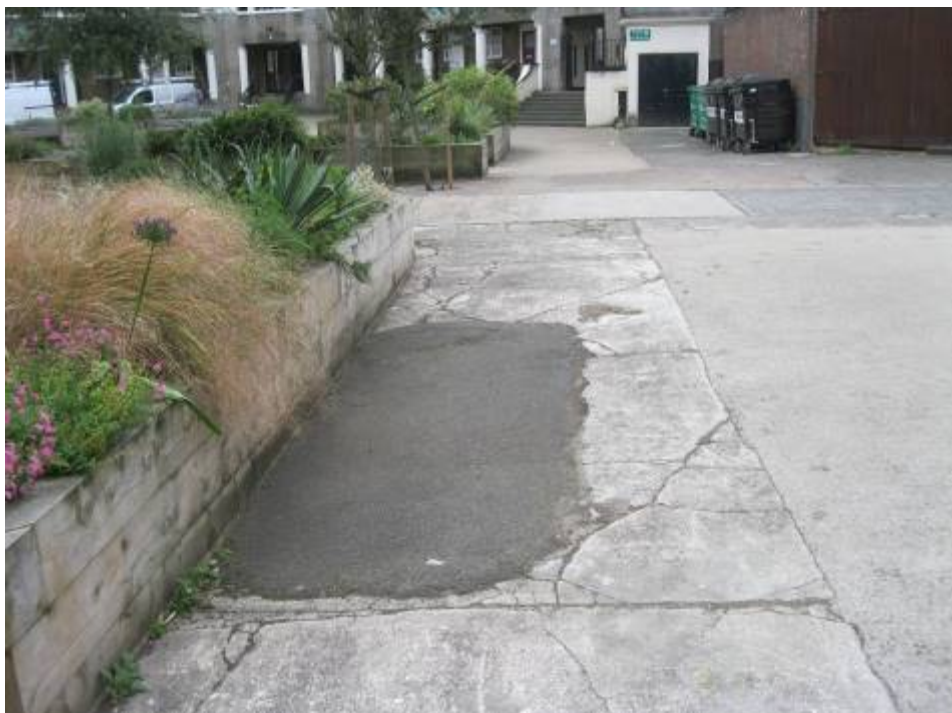
Photograph 40 Courtyard typical paving condition
