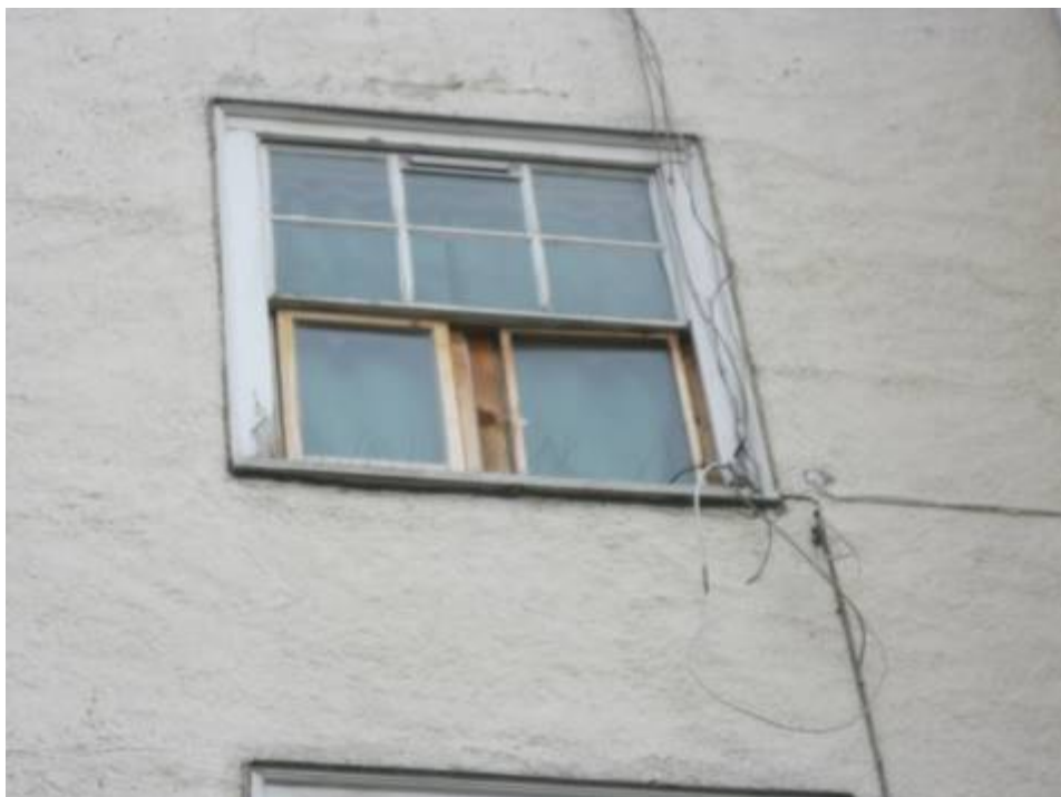
Photograph 30 Improper alteration to window
