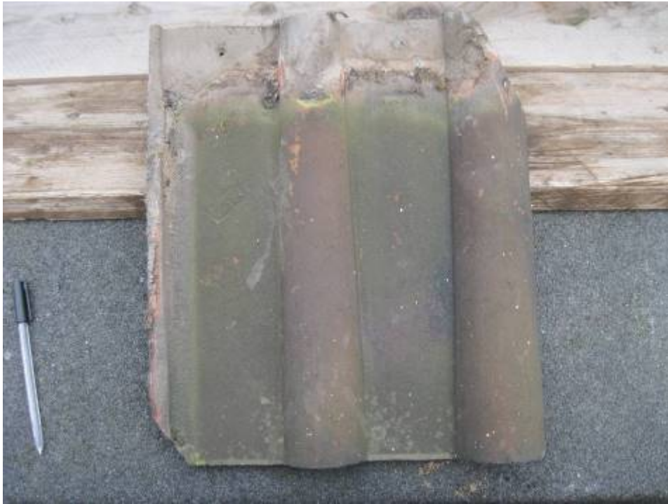
Photograph 11 Existing tile condition
