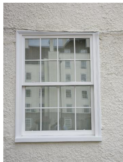
Principal of proposed replacement timber window type as fitted in adjacent part of Levita House but with semi-concealed sash balances
