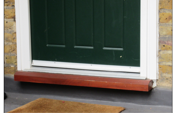
Rebated door panel detail Note: Photo to illustrate panel detail only Hardwood cill is not part of this application
