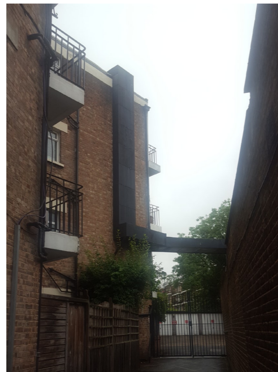
View North from access road of ducting running up 134-141 Cholmley Gardens
