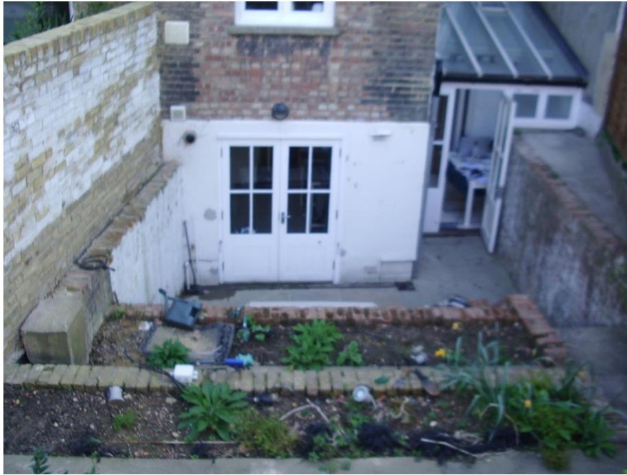
The rear elevation of no. 9, St George's Terrace at basement level as existing showing the impact of the excavation of the original garden to create three terraces stepping down to basement level
