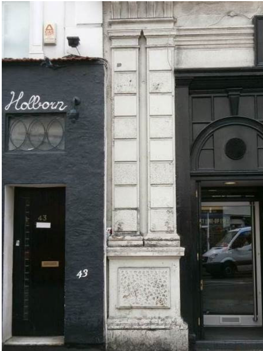
Front Elevation – Ground Floor – flaking decoration and sub-fluorescence to plinth. Paint-obscured vermiculated render panels.
