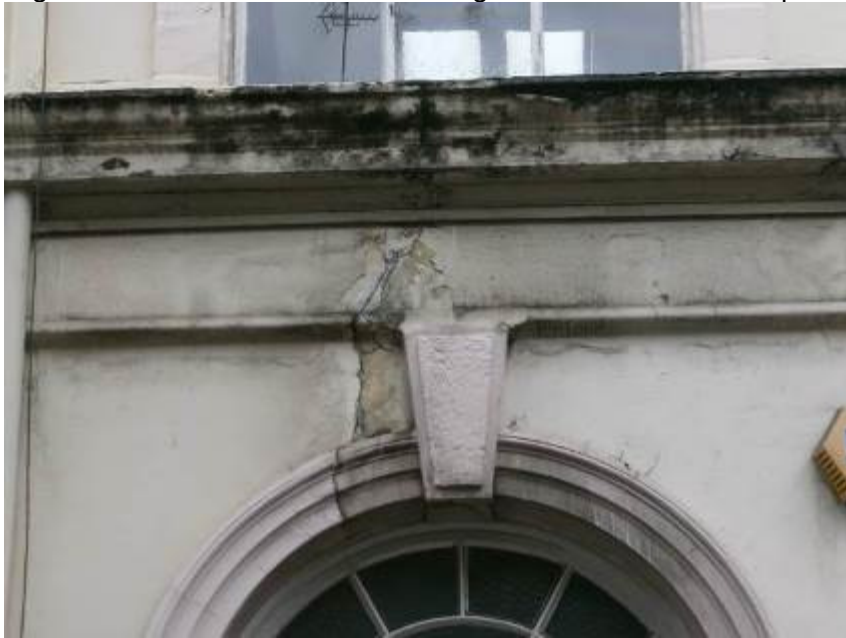
Right Hand Side Elevation – cracking to window heads and plinth. Flaking decorations.
